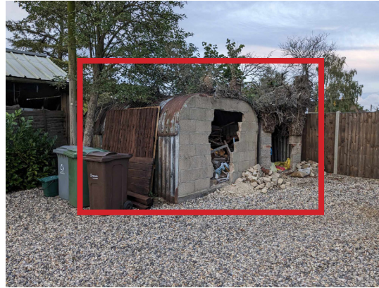
IMAGE OF THE 2 SHEDS, NEIGHBOURS OUTBUILDING IN VIEW ON THE LEFT, TREES WILL BE REMOVED.
