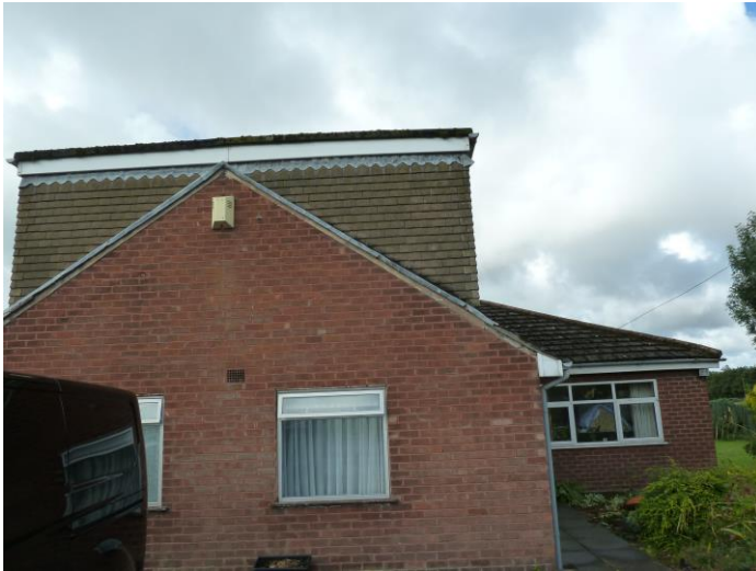
Photograph 9: B1 – typical view of the east (side) elevation showing dormers and lead flashing at verge.
