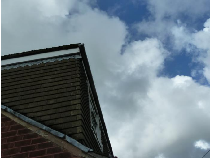
Photograph 11: B1 – east elevation note gaps behind flashing on dormer at verge.
