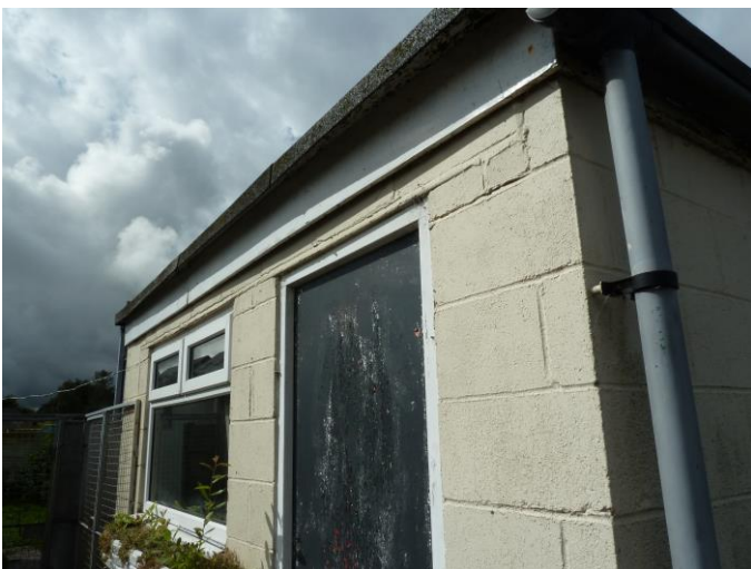
Photograph 19: B5 – typical view – concrete block construction. Gap at fascia very shallow and exposed. No PRFs.
