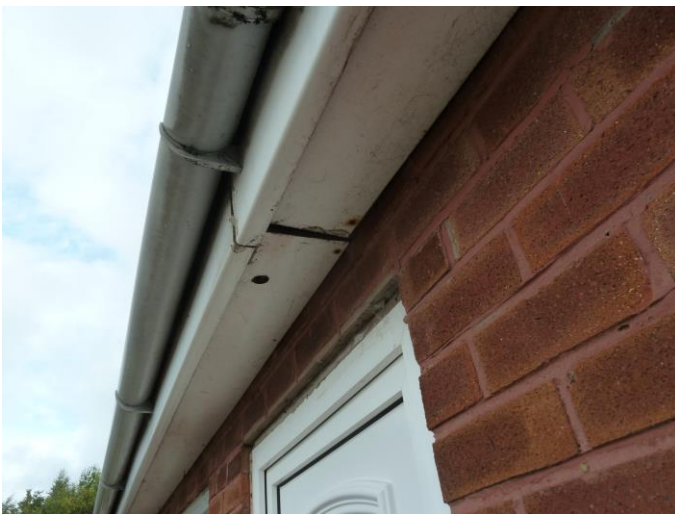
Photograph 13: B1 – west elevation – gaps between panels below soffit allow access to PRFs in soffit and possibly roof.
