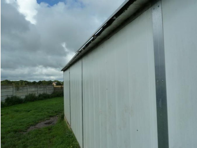
Photograph 17: B4 – typical view – modern modular kennel block with runs - no PRFs.
