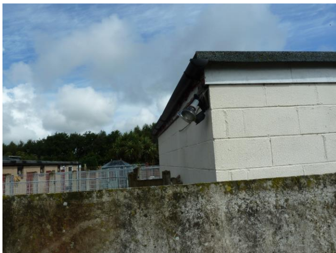
Photograph 20: B5 – typical view – concrete block construction. Gap at fascia very shallow and exposed. No PRFs.
