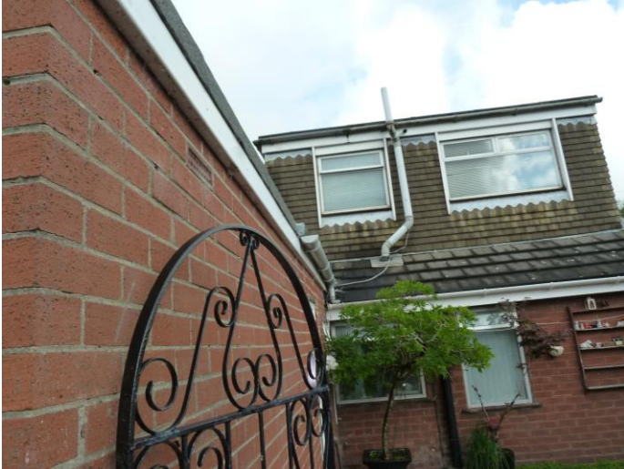
Photograph 8: B1 – typical view of the rear dormer and single-storey rear extension. Note tight-fitting UPVC fascia board.
