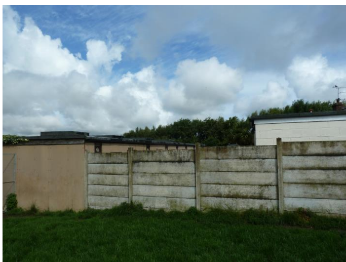
Photograph 21: B6 – typical view – south and east elevations of pre-fab kennel block. No gaps at fascia. No PRFs.
