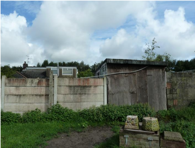
Photograph 15: B3 – typical view – pent felt roofed with single skin board construction and no PRFs.
