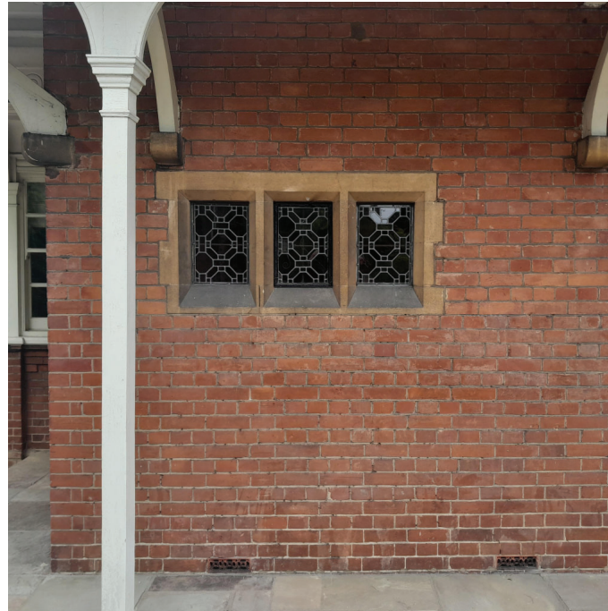
Existing leaded window and stone surround to be removed and installed where existing EDG08 is currently located
