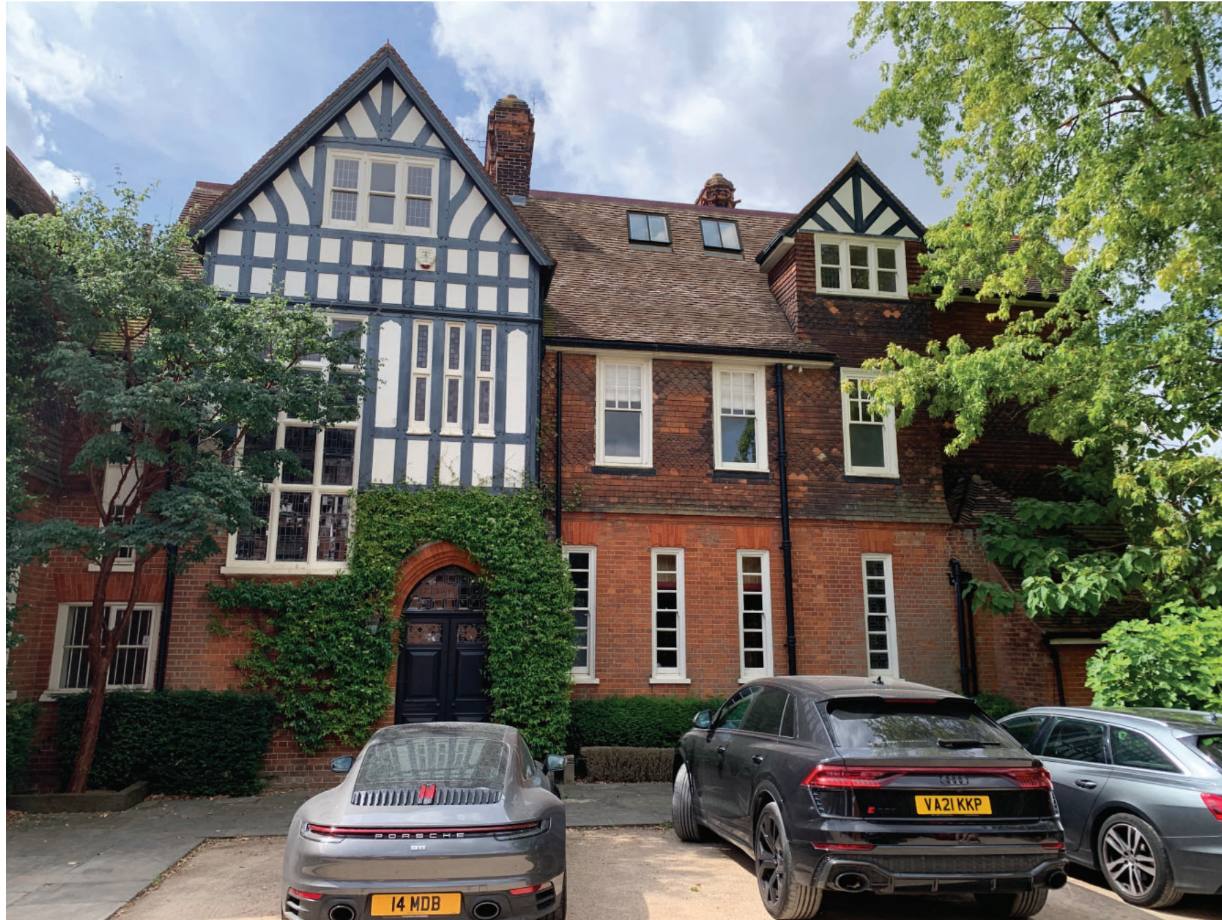
Image of North elevation showing the altered roof following the removal of the existing dormer window
