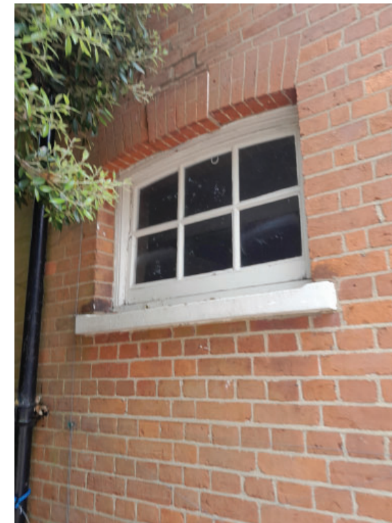
Existing window with slipped arched lintel
