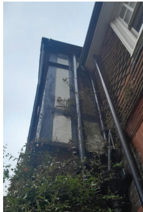
Existing damaged render to be replaced
