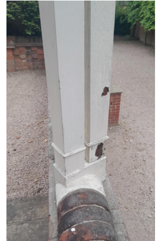
Rotten timber column to garden veranda
