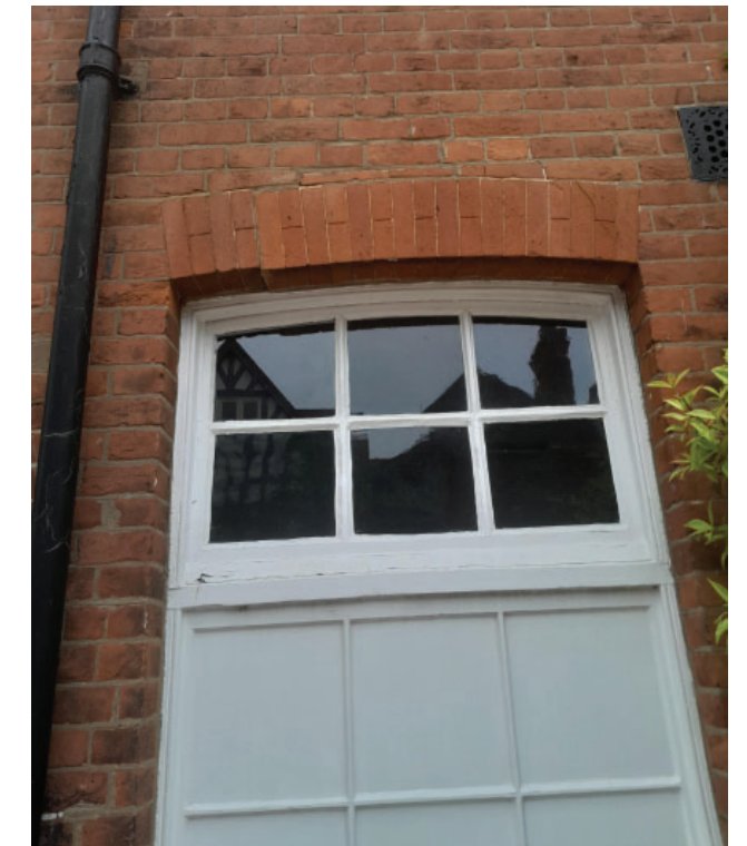
Existing window with slipped arched lintel and cracked brickwork
