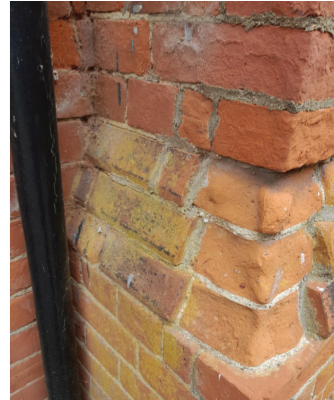
Image showing area of erroded brick work to be replaced
