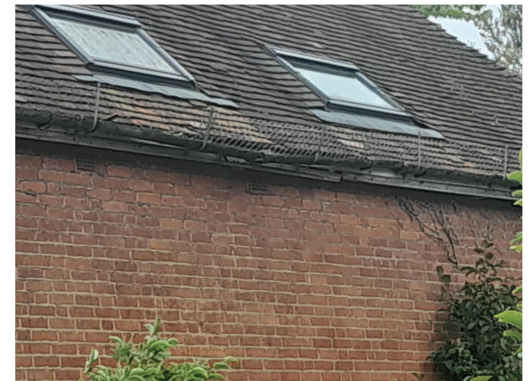
Broken gutter to the coach house will be repaired
