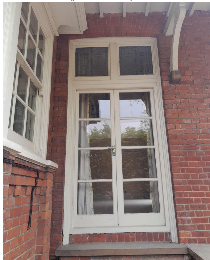
Existing glazed timber framed door and top light to be removed and installed where existing Window WG32 is currently located
