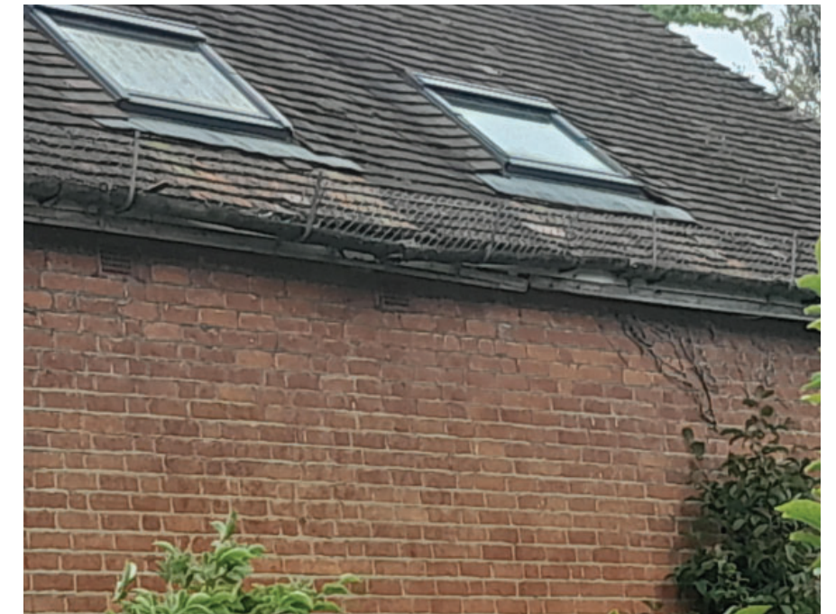
Broken gutter to the coach house will be repaired
