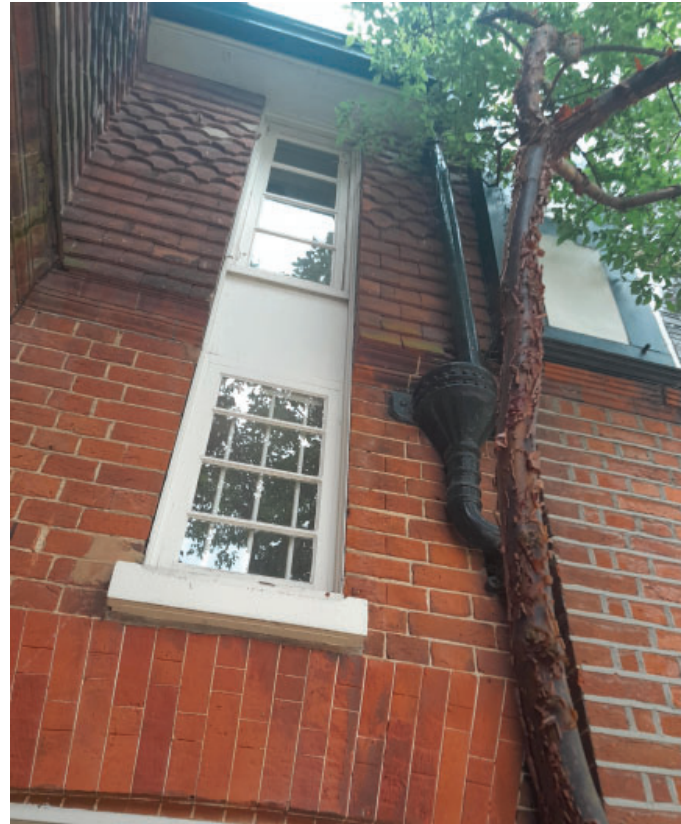
Image of North elevation showing cement pointing and concrete repairs to the clay tiles
