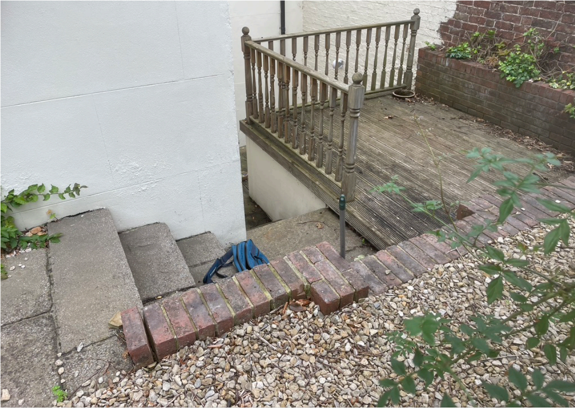
Picture of modern steps to be revised to allow for proposed extension
