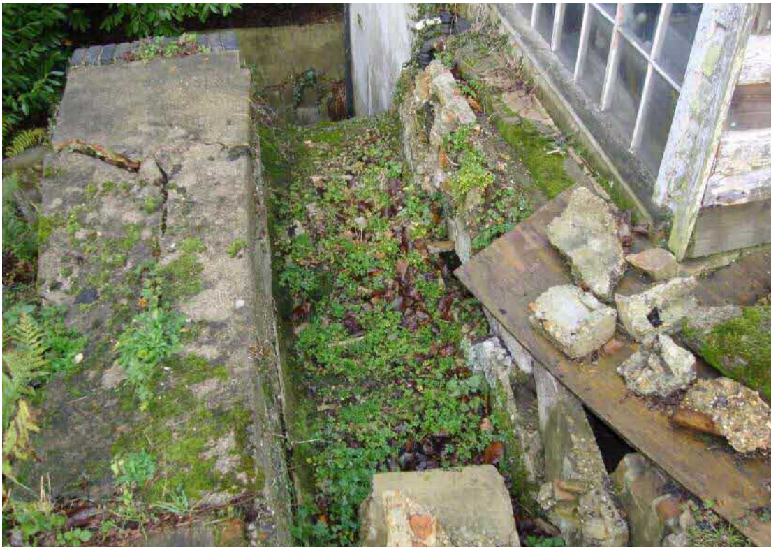
Fig.52 ‘Significant voiding’ has occurred under the building
