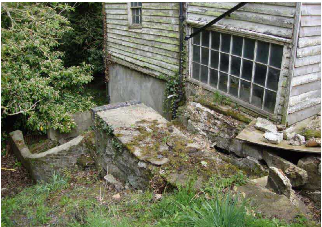
Fig.51 Suffering from 'slow decay' with 'no solution agreed'
