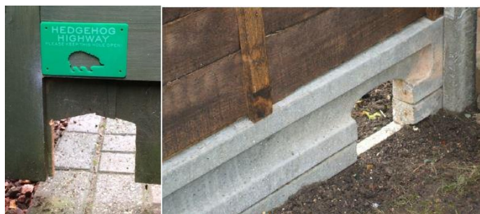
Insert 3: Showing wildlife access gap within fencing
