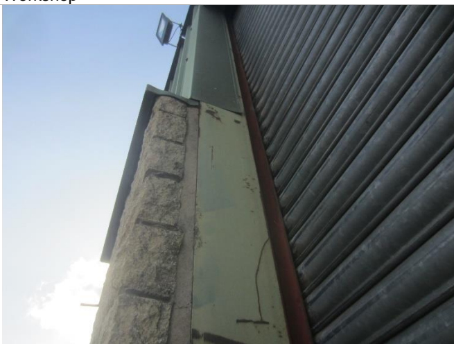
Photo 17: Sealed mortar at roller doors of Building 1 (with gap at the top of the door)
