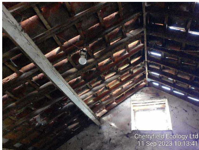
Figure 22- Gaps between rafters and wall plate of B1a.
