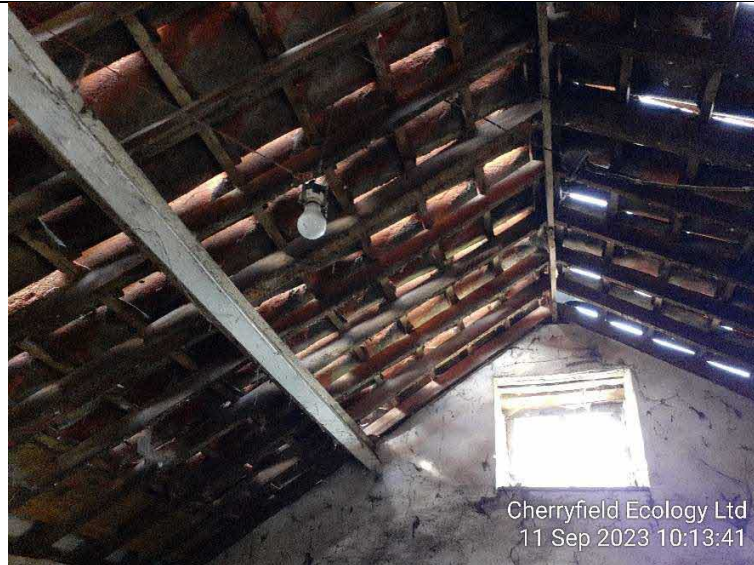
Figure 6- Ceiling with exposed tiles.
