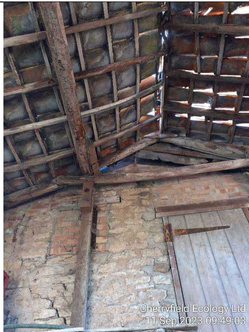
Figure 21- Cracks within the brickwork of B1b.
