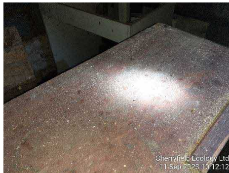
Figure 20- Urine staining within B1a indicating bat presence.
