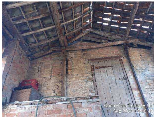
Figure 9- Rafters and joists in poor condition across the roof of the building.
