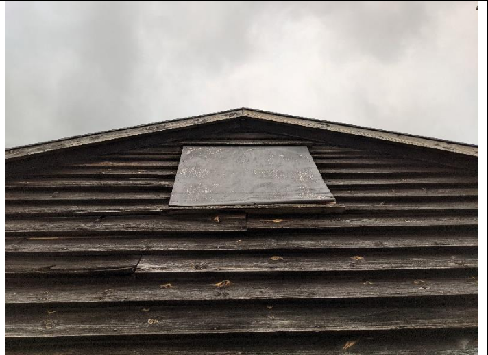
Photo 8 Warped weatherboarding on west gable end of barn with bat roosting potential
