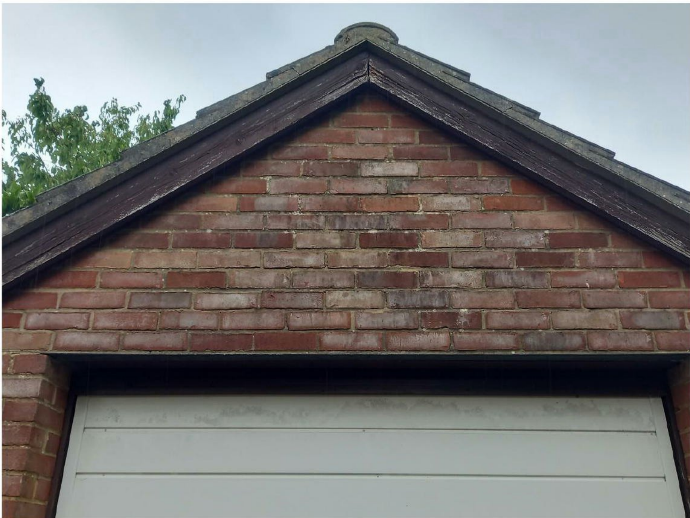
Plate 8 – Southern aspect of building 2, showing some gaps around the gable end.
