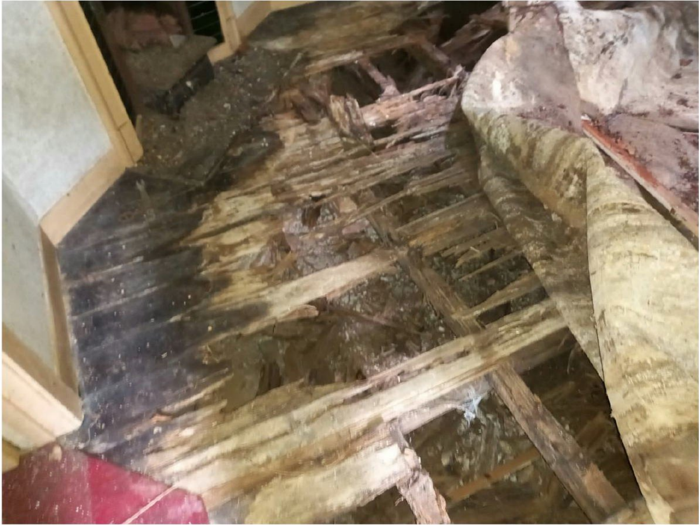
Plate 19 – Internal photograph of building 4, showing heavy damage to structure.
