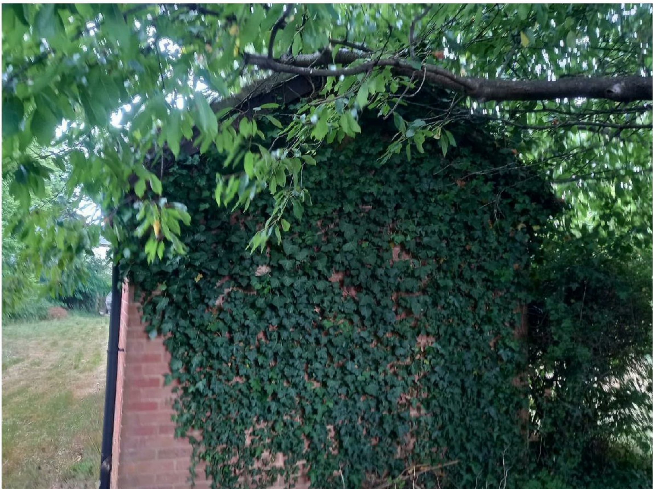
Plate 10 – Northern aspect of building 2, showing heavy ivy growth.
