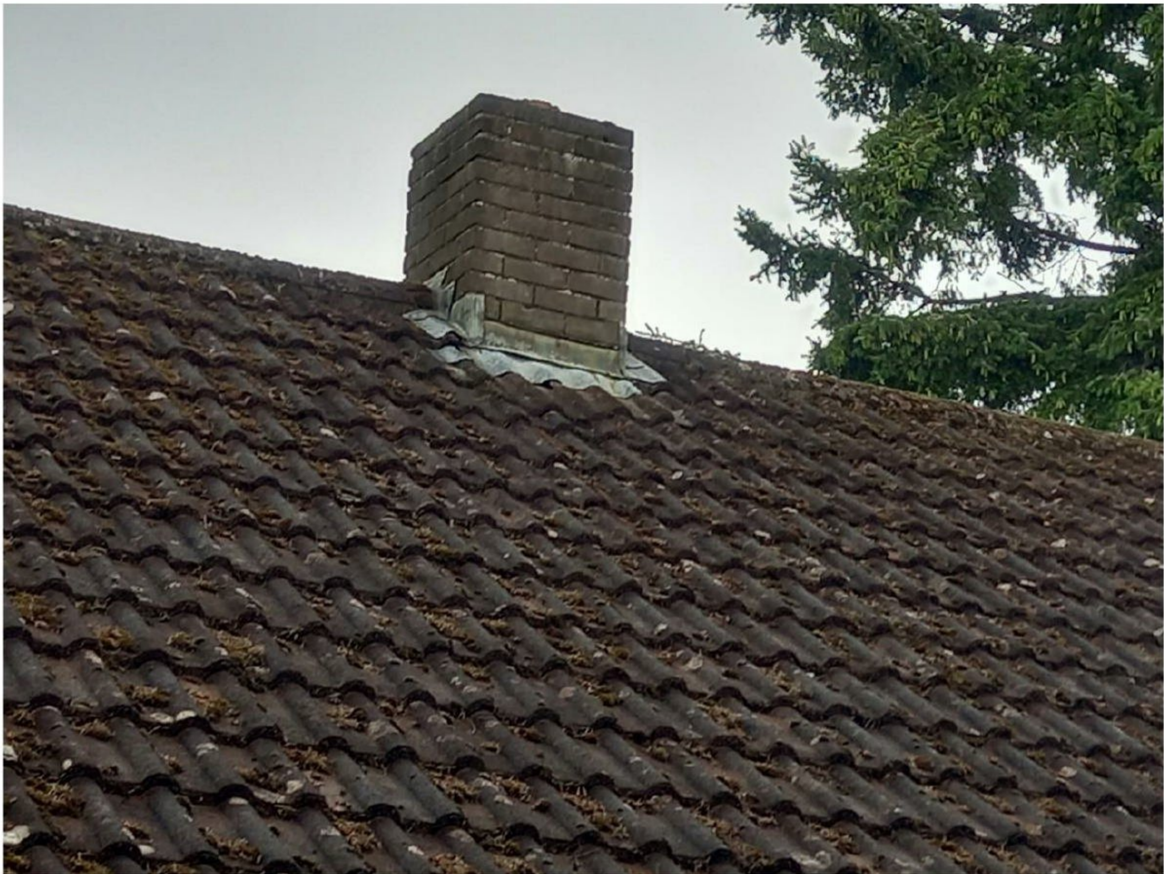
Plate 5 –Roof of building 1, showing gaps underneath lifted lead surrounding the chimney.
