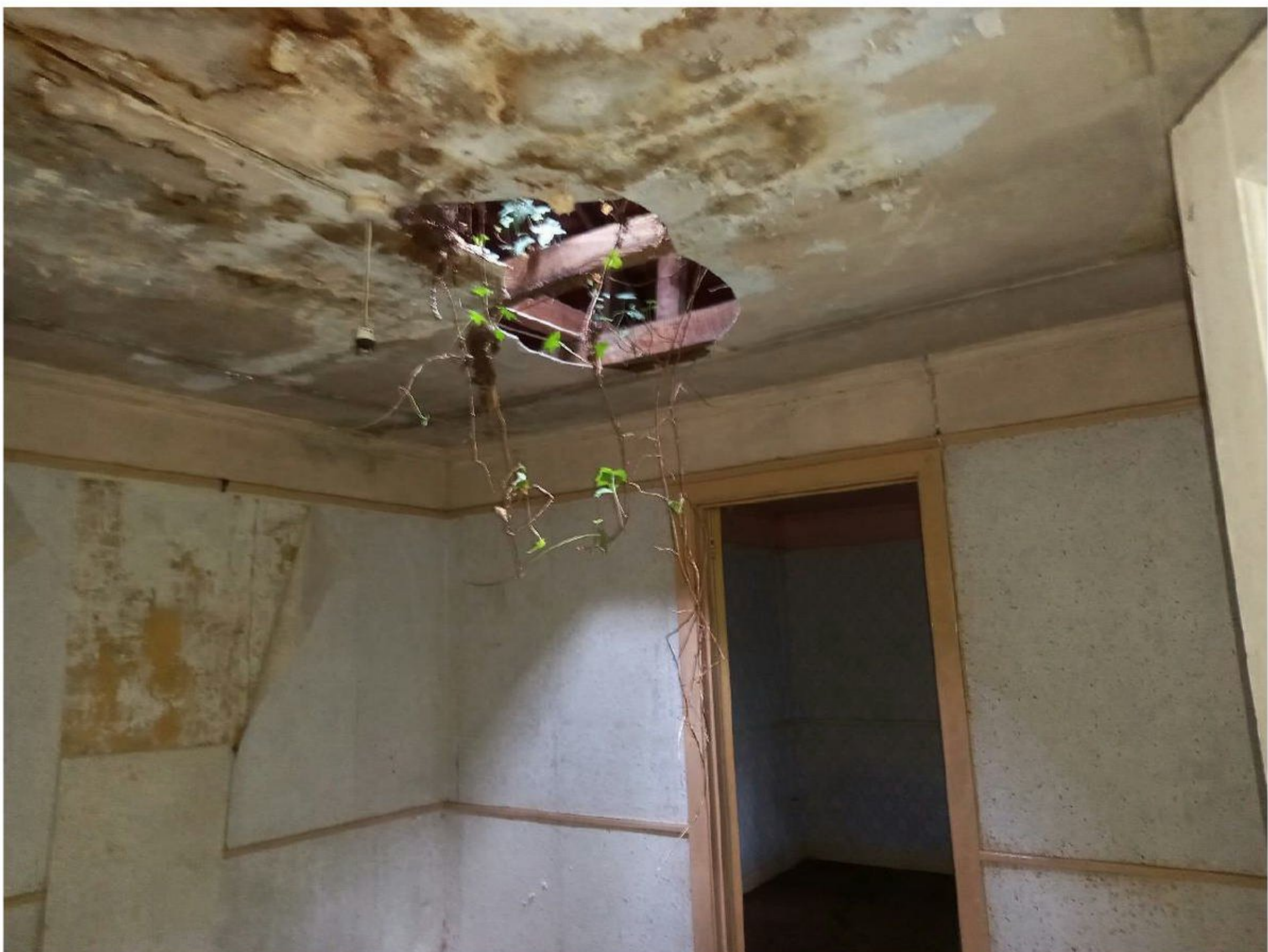
Plate 18 – Internal photograph of building 4, showing heavy damage to structure.
