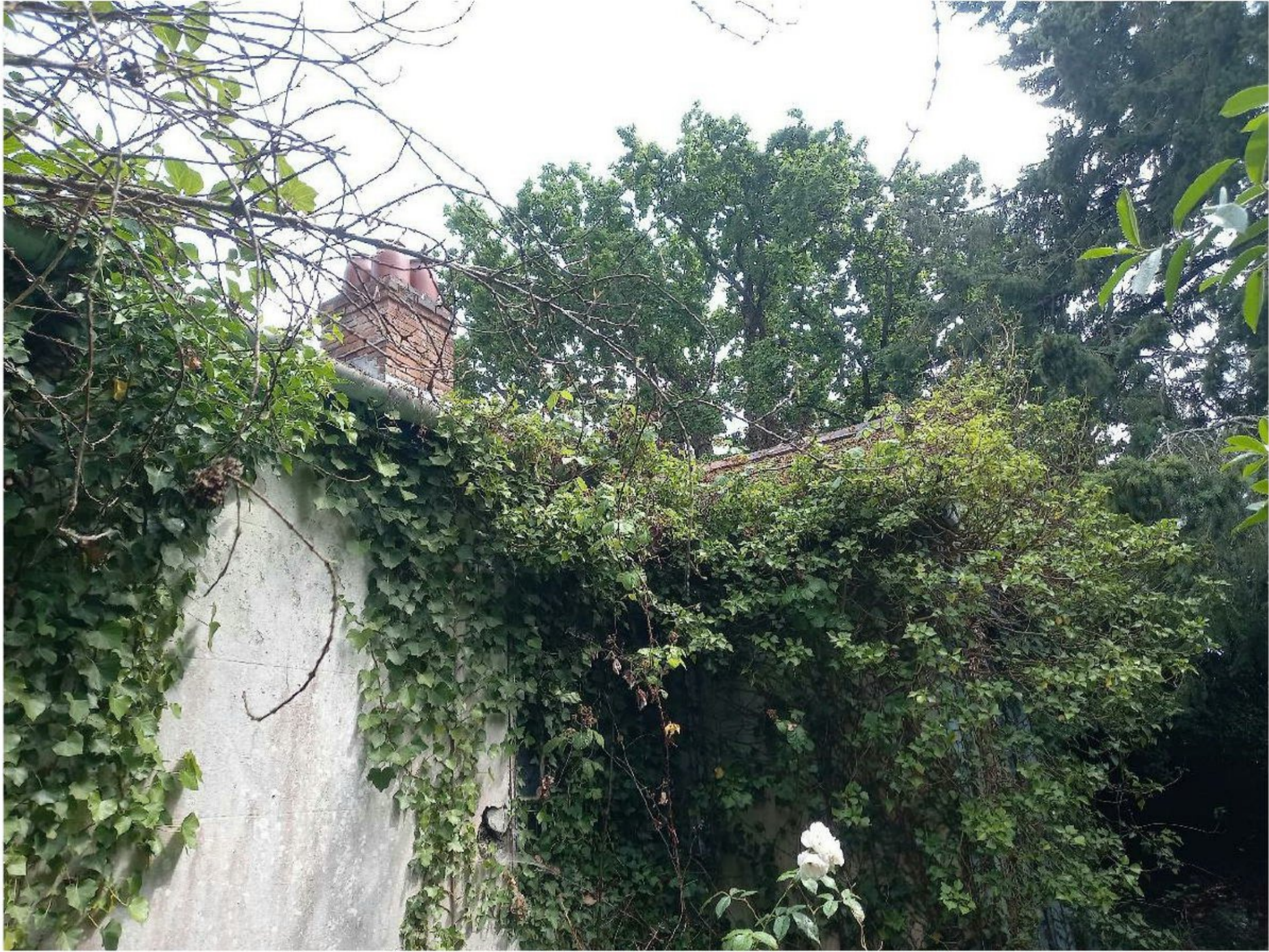
Plate 17 – Eastern aspect of building 4, showing cracks in wall and heavy overgrowth.
