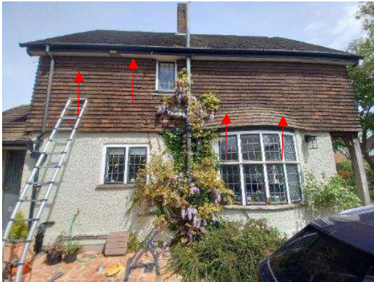
Photo 14: West elevation – gaps at eaves, under hanging tiles around bay window and where tiles forced apart by climbing vegetation (in the past)
