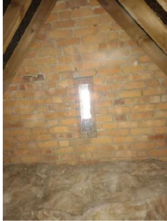
Photo 6: East end of subservient east-west loft with ventilation slit in gable wall
