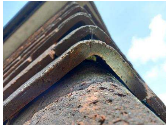
Photo 13: Gaps between 'corner' hanging tiles (all elevations)
