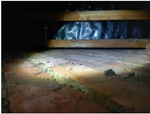
Photo 17: Chimney breast with bat droppings indicating potential access point (TN3)
