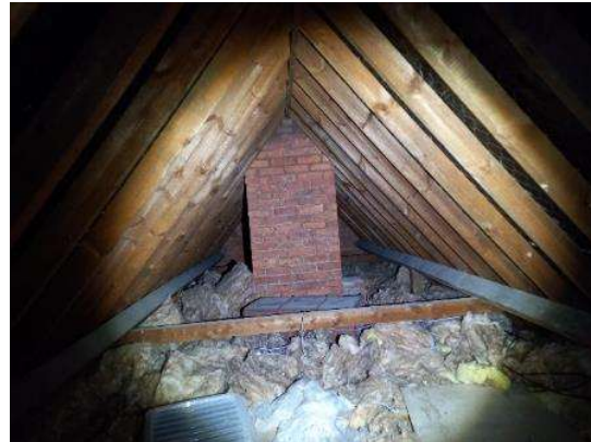
Photo 8: Looking towards east end of subservient east-west loft with chimney breast in foreground
