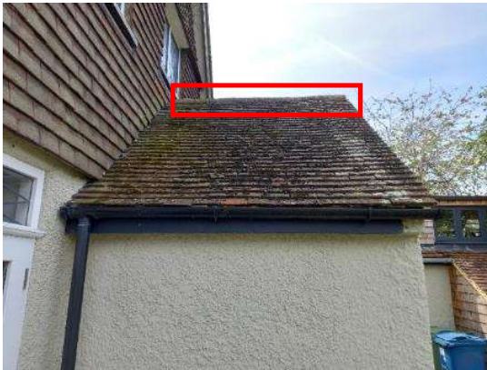
Photo 12: Missing mortar/gaps under ridge tiles on rear single-storey extension
