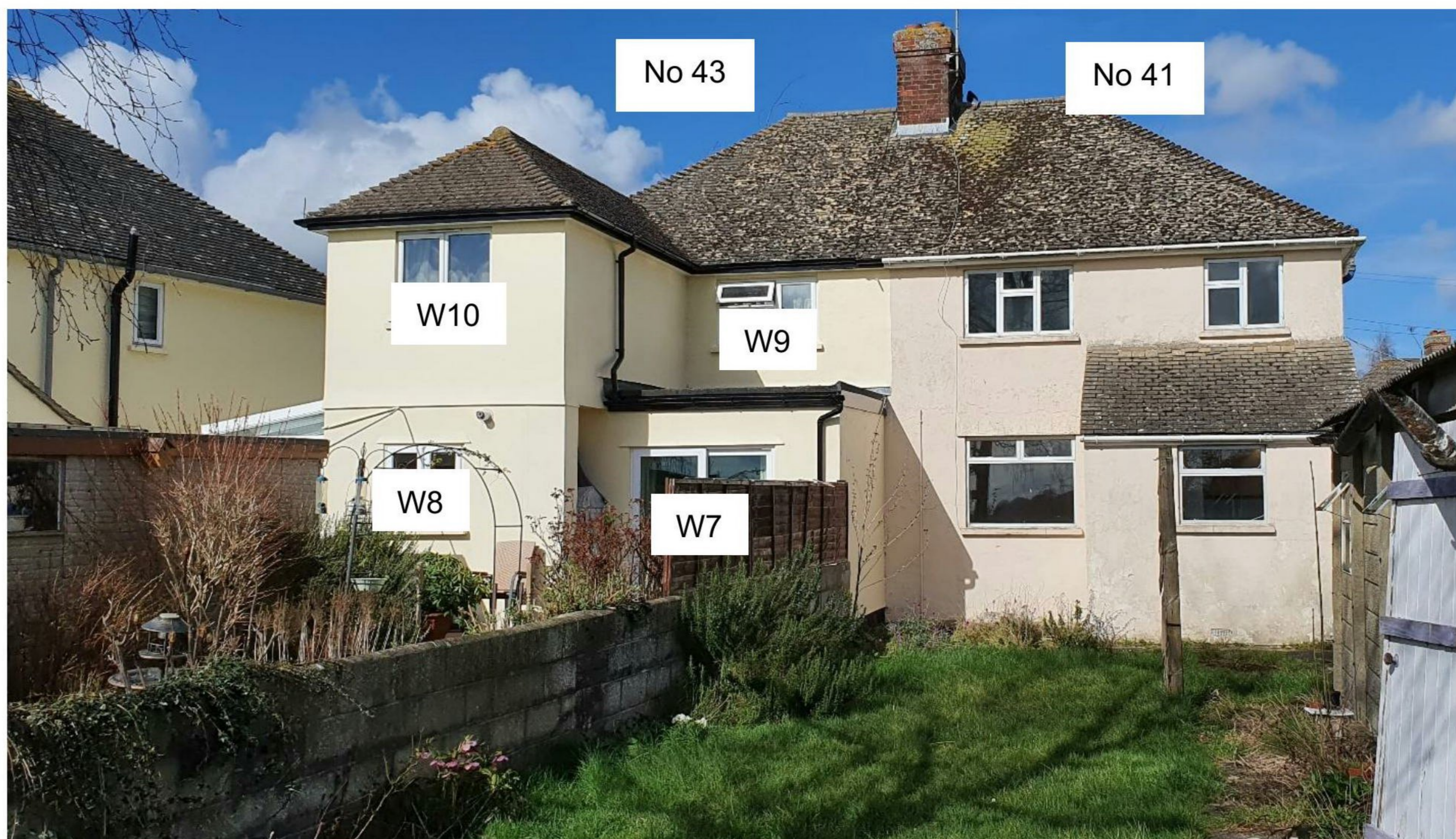
Figure 3 Photograph (taken during site visit) showing the analysed windows at 43 Meadow Prospect, labelled W7 to W10.
