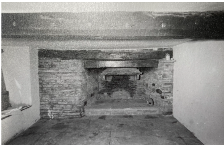
Dining room in 1972, before the oven was revealed, with original slab floor
