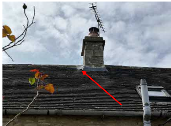
6: Gap under lead flashing.
