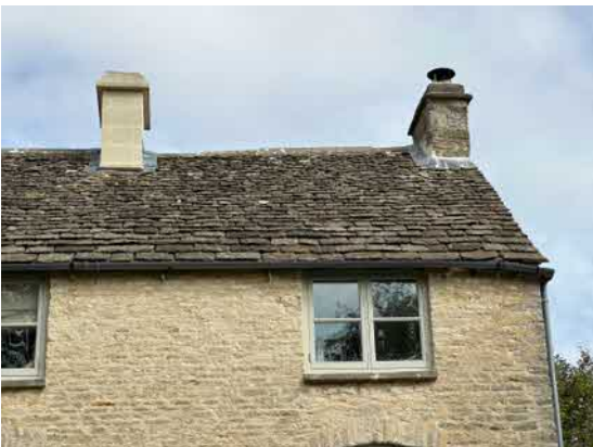
5: Gaps under slates on the south roof slope.
