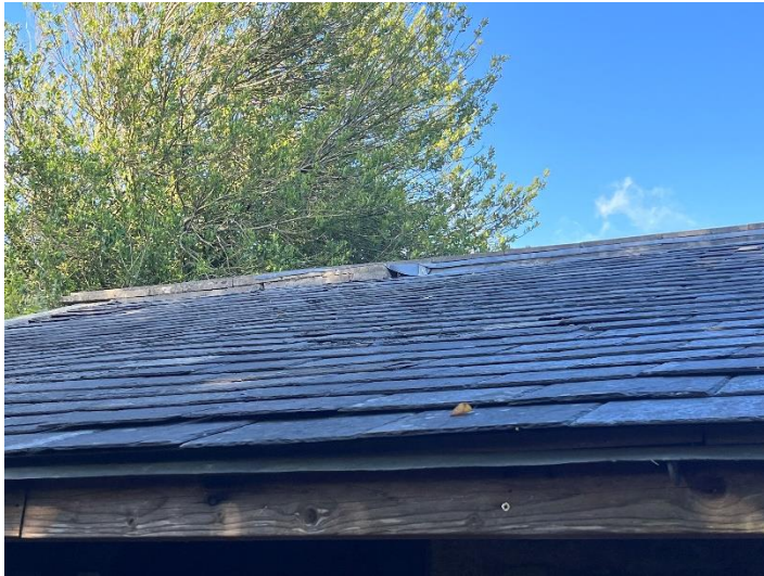
Figure 3: Raised tiles and gap beneath lead flashing at the northern end of the building
