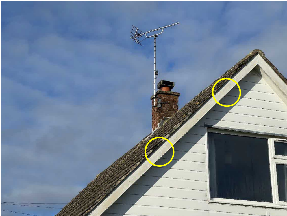
Photograph 5: The eastern tile crease with missing mortar.
