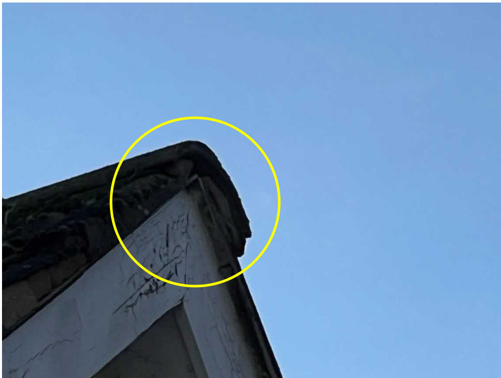
Photograph 6: The ridge tile with missing mortar at the western gable end.
