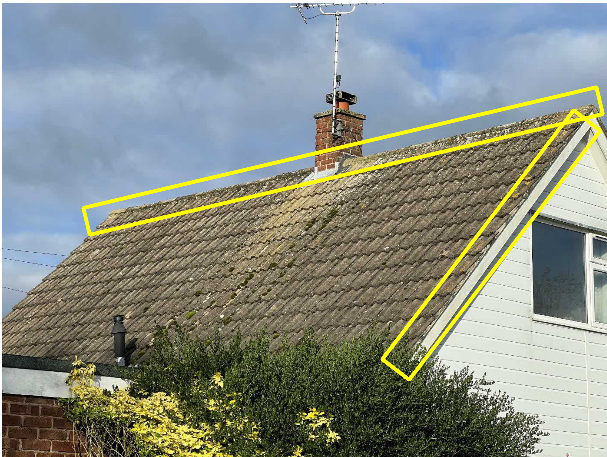
Photograph 7: The areas of the roof to be stripped (highlighted in yellow) under the supervision of a licenced bat ecologist.
