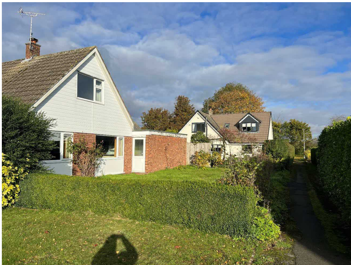
Photograph 3: The south aspect of the roof and east elevation of the building.
