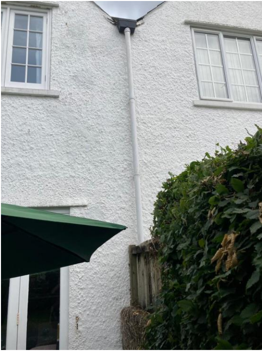
Boundary at rear. The centre of the downpipe aligns with the boundary. The fence and wall are on the applicant's property.
