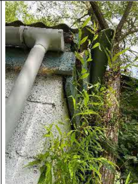
Figure 10 Lifted fascia on the south-eastern elevation.
