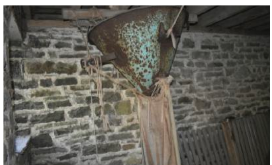
Fig.16. Grain shoot from granary (barn 1) into trap house area (barn 2)
