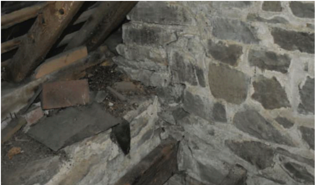
Fig.27. Internal first floor wall (between barns 3 and 4) butting up against western elevation of barn 4 at eaves level.
