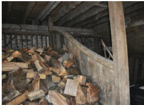
Fig.13. The ground floor interior of Barn 1 with pony stalls and hay racks
