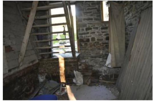
Fig.19. Interior of trap house with partially submerged floor and steep timber ladder stair
