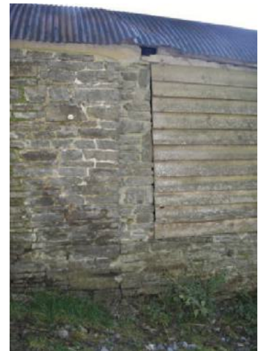
Fig.36. Straight joint between barns 5 and 6 on the north wall
