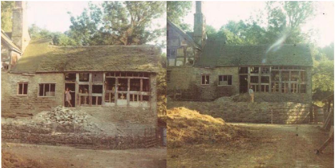
Fig.40. Scans of photographs from 1972 showing the construction of the wall at the south end of the courtyard in progress.
