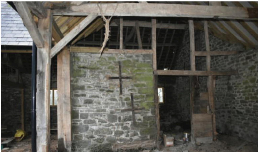
Fig.28. Free standing wall in barn 4, on possible line of earlier configuration and showing good, possibly later, quoins but poor original wall construction
