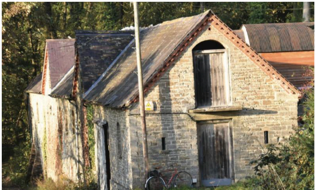
Fig.12. South facing elevation of Barn 1 and part of the west facing elevations of barns 1, 2 and 3
