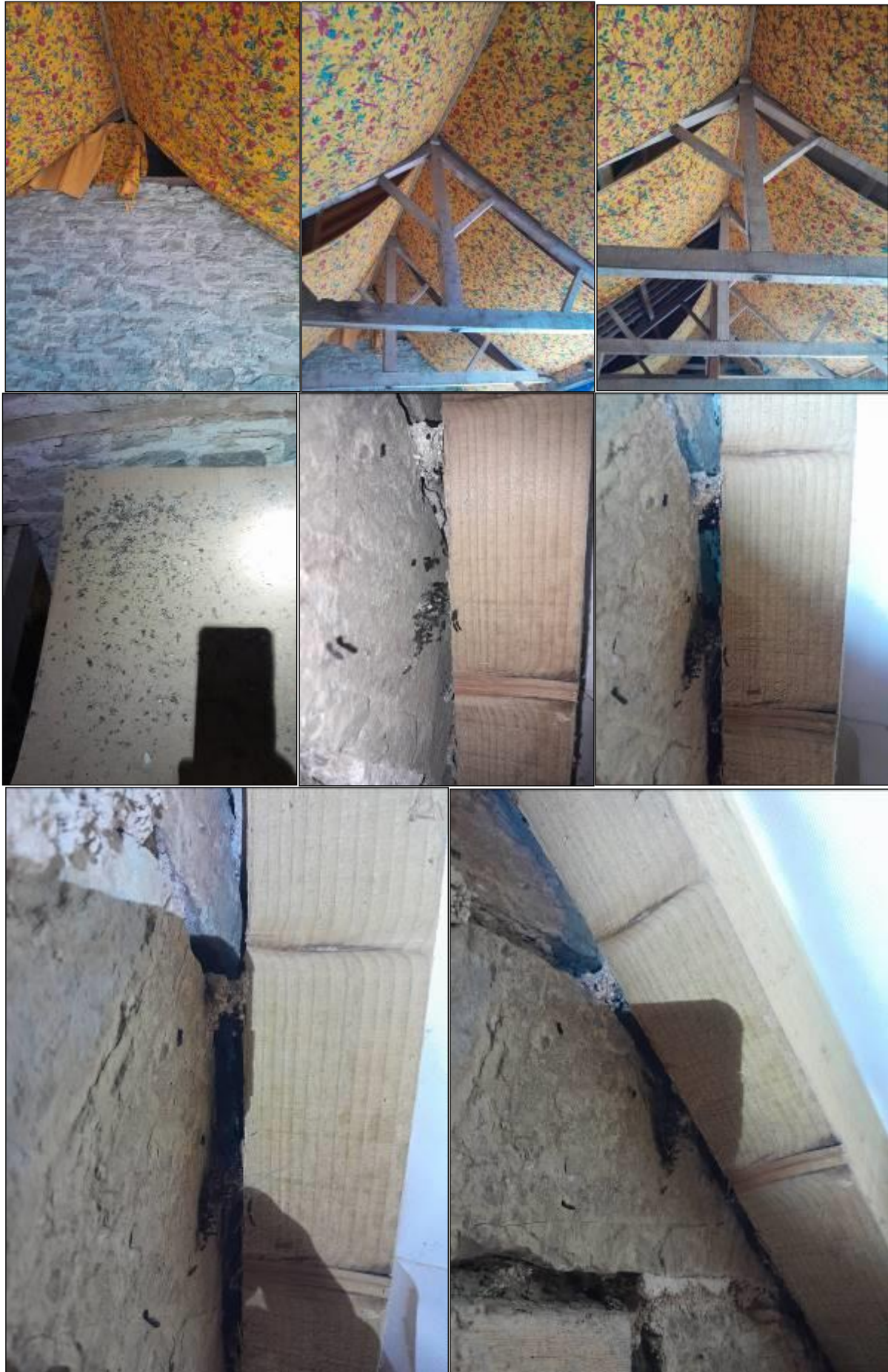
Additional interior images showing the droppings within the Barns .
