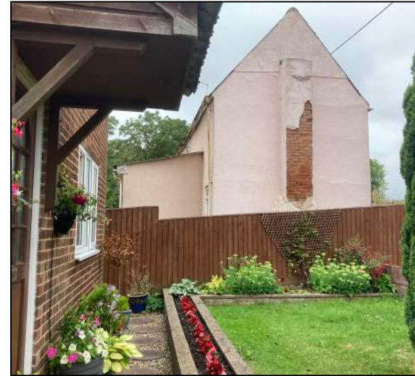
Figure 7: East gable of existing house seen from the front of the neighbouring building, Aronoel
