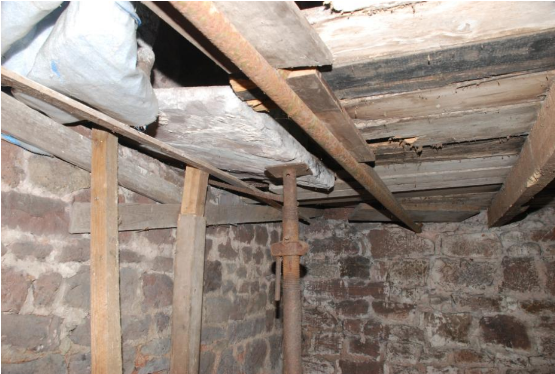
Plate 32: Cider Mill GF Cider House temporary propping to first floor showing underside of hearth stone.
