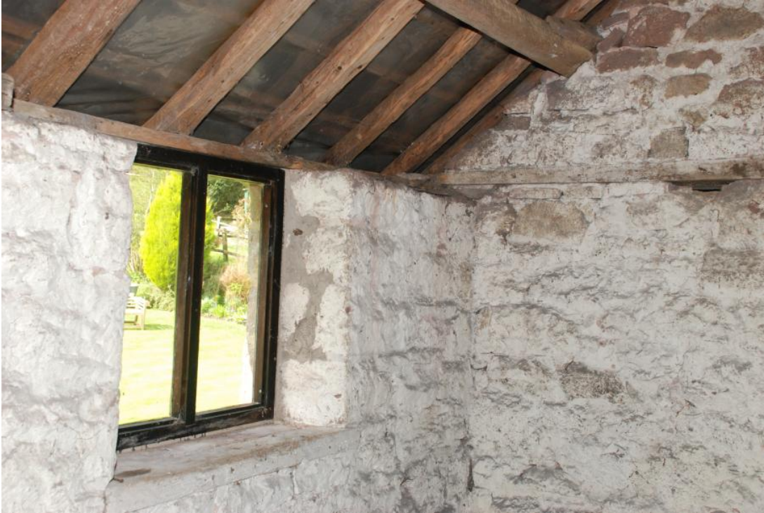
Plate 20: Cider Mill FF loft detail of south west corner showing window, part roof and timber wall ties.
