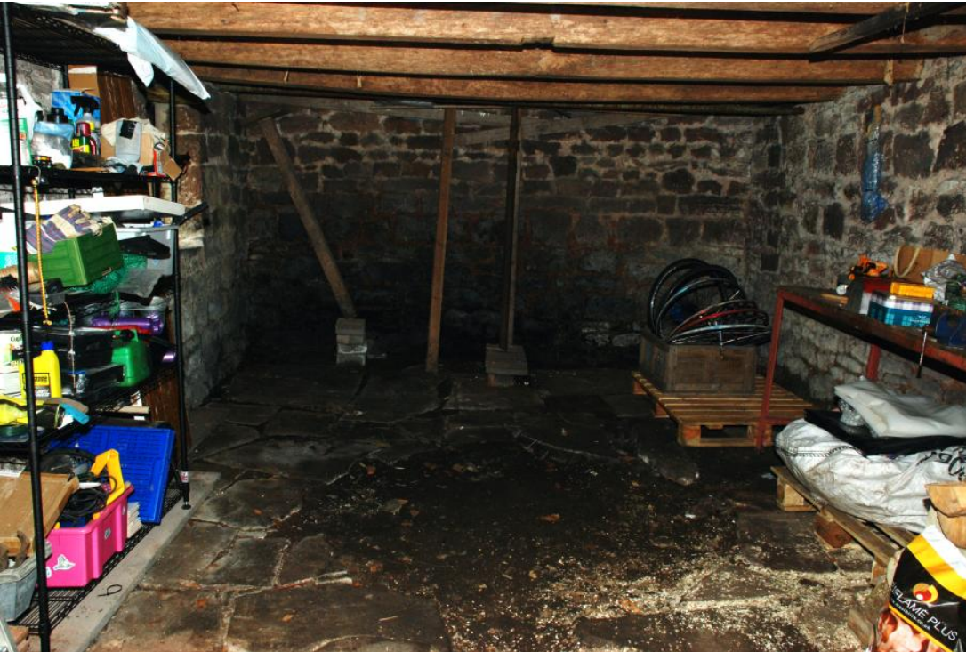
Plate 26: Cider Mill GF Cider House general interior view to west.
