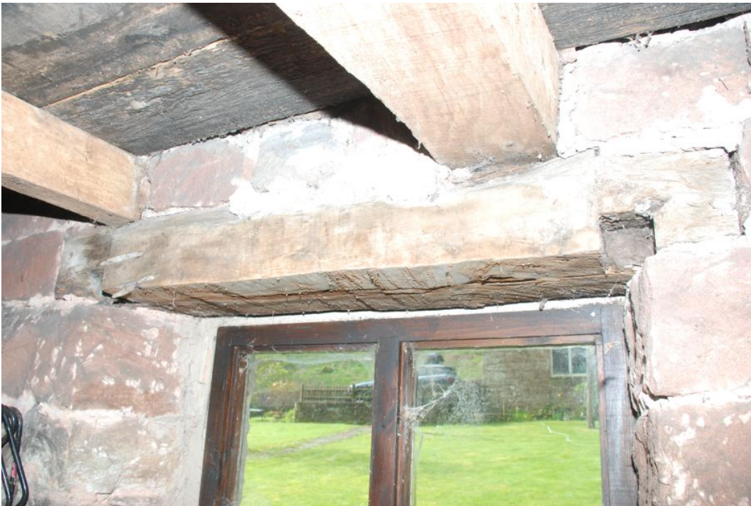
Plate 33: Cider Mill GF Cider House detail of first floor beams and window lintel.
