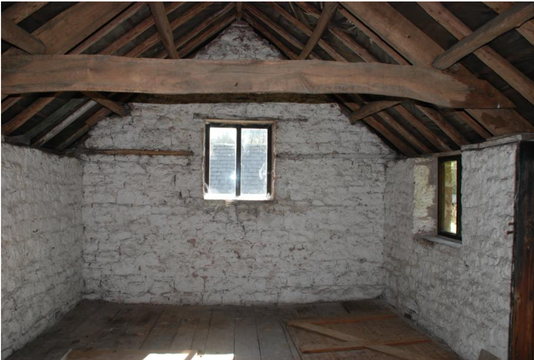
Plate 17: Cider Mill FF loft general interior view to east showing roof structure.
