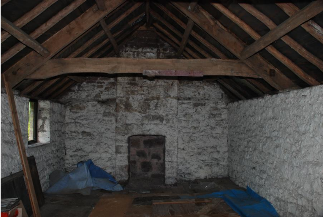
Plate 18: Cider Mill FF loft general interior view to west showing fire place and roof structure.
