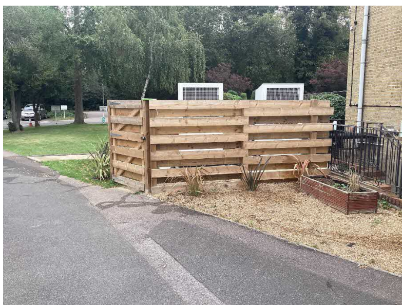
Figure 2: View of the ASHPs looking towards the northeast, enclosed by timber fencing and phormium planting, expected to grow to approximately 2ft 6in (76 cm).
