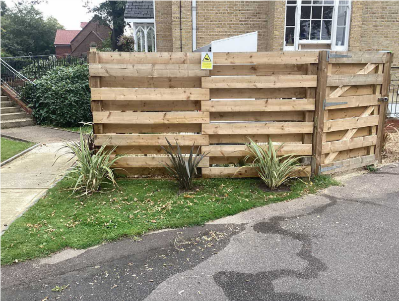
Figure 3: View of the ASHPs looking towards the southeast, enclosed by timber fencing and phormium planting, expected to grow to approximately 2ft 6in (76 cm).
