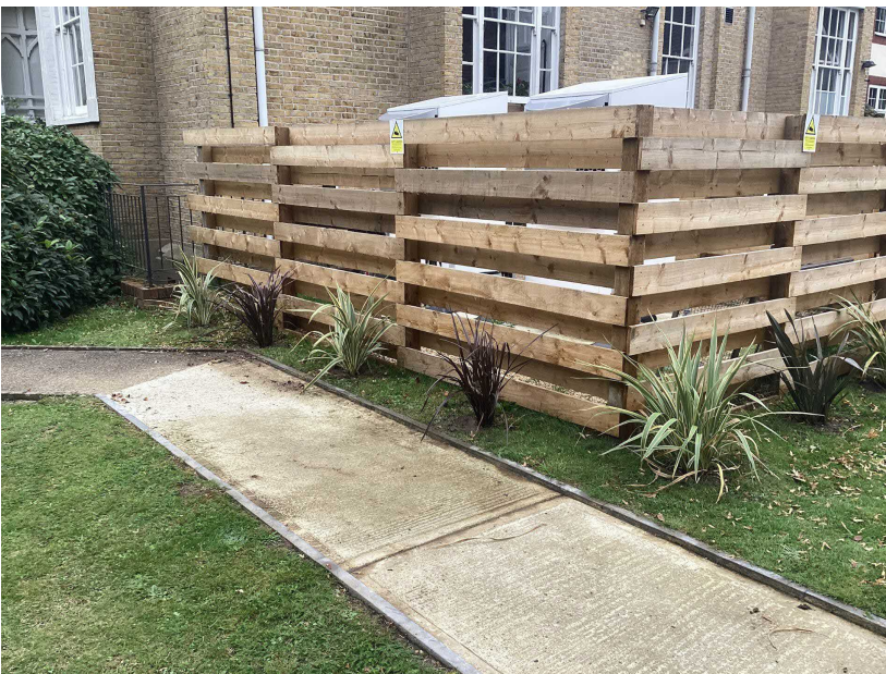
Figure 4: View of the ASHPs looking towards the south, enclosed by timber fencing and phormium planting, expected to grow to approximately 2ft 6in (76 cm).
