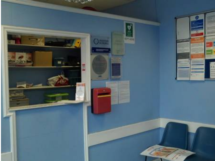
Inside the existing dental surgery waiting area. This will be converted to a studio flat.
