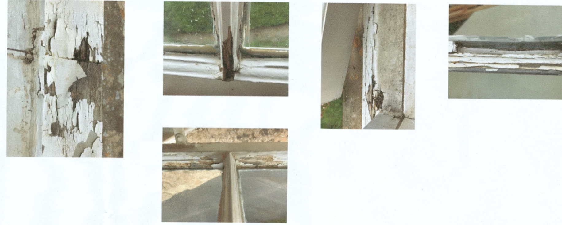
Various views of defective & rotten frames.
