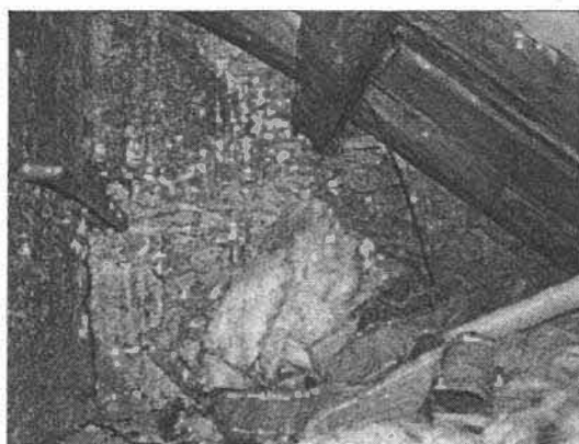
Plate 27: Upper part of the roof structure looking west (above) and east (right)
