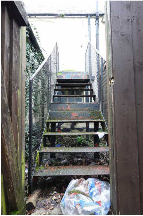
Figure 6 – existing fire exit and secondary access to the current residential accommodation on the first floor. This is proposal is to replace with a oak type stair case and access to the first floor.
