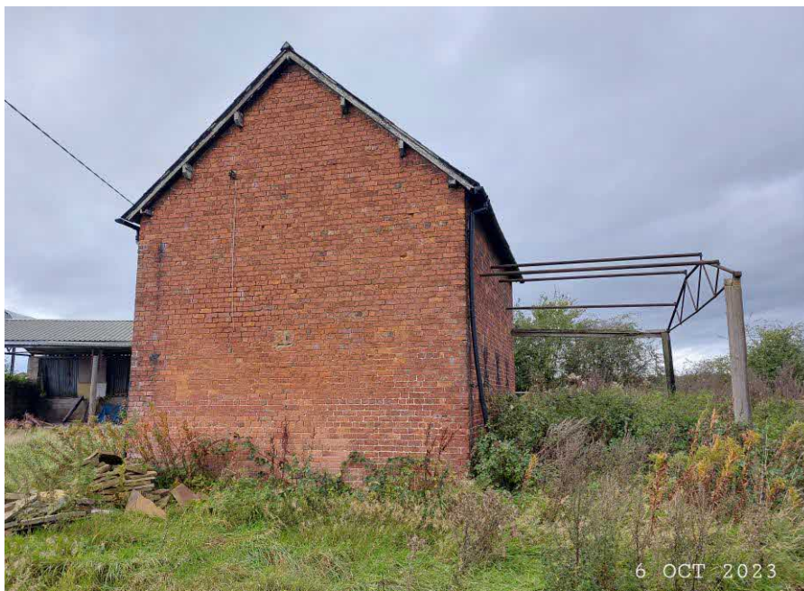
Figure 1: Photo taken at Manor Farm on the 6 th of October 2023, before the commencement works began.
