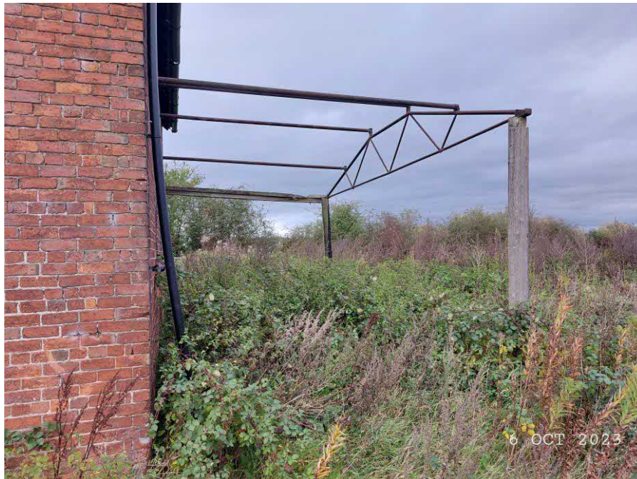
Figure 3 – Photo taken at Manor Farm depicting the site before commencement began on the 6 th of October 2023.
