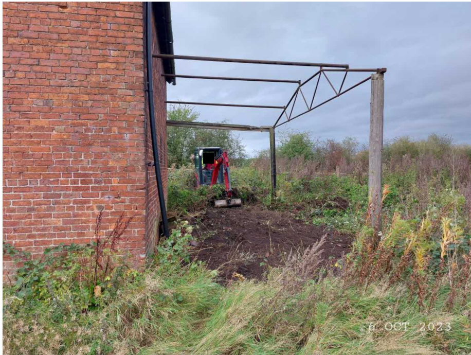
Figure 4 – Showing the beginning of the commencement works on the 6 th of October 2023.
