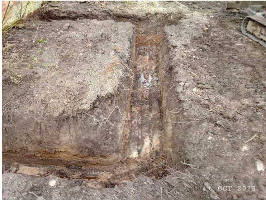
Figure 10 – The footings dug out at the Coach House during commencement works on October 6 th ,2023.
