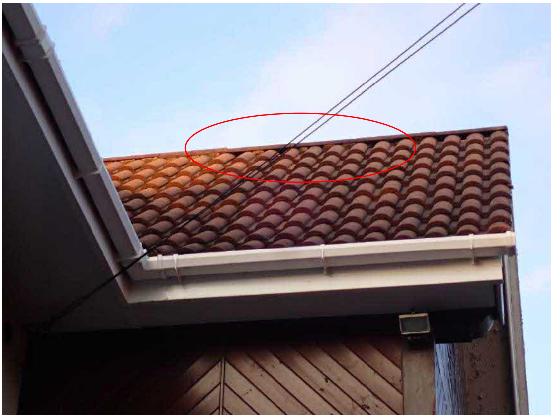
Photograph 6 – gaps due to the missing mortar under the ridge tiles on the western aspect.
