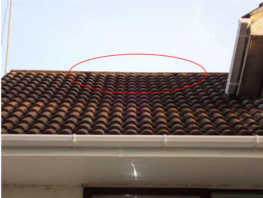
Photograph 5 – gaps due to missing mortar under the ridge tiles on the northern aspect.
