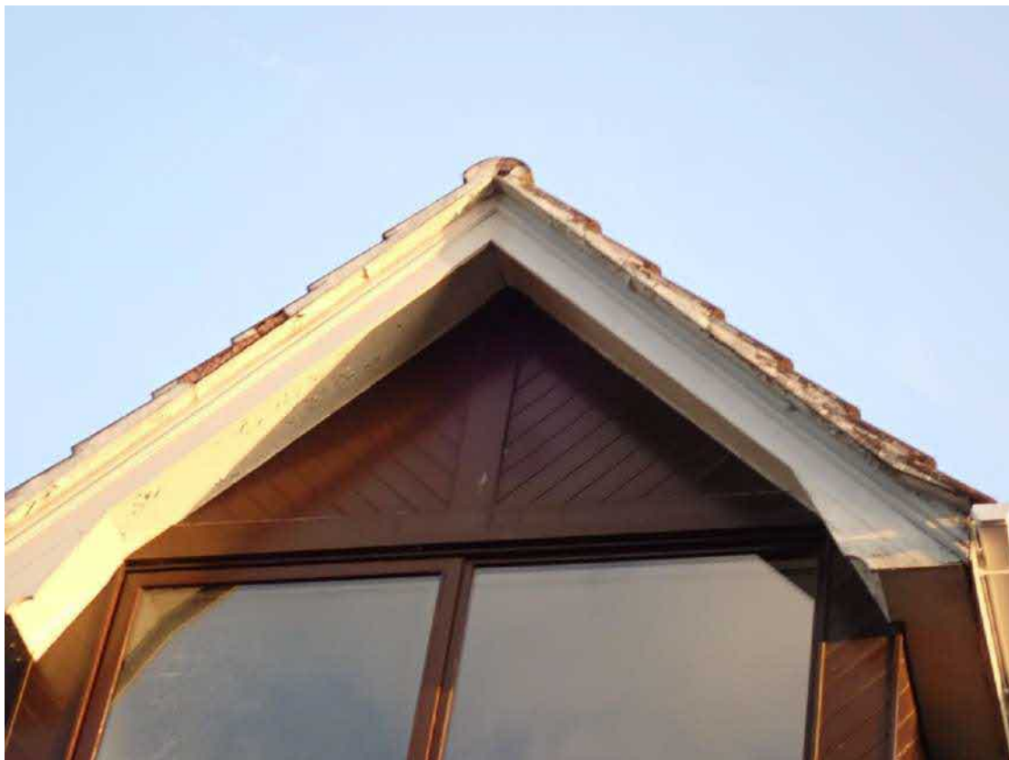
Photograph 8 – missing mortar at the apex of the dormer window on the rear elevation.
