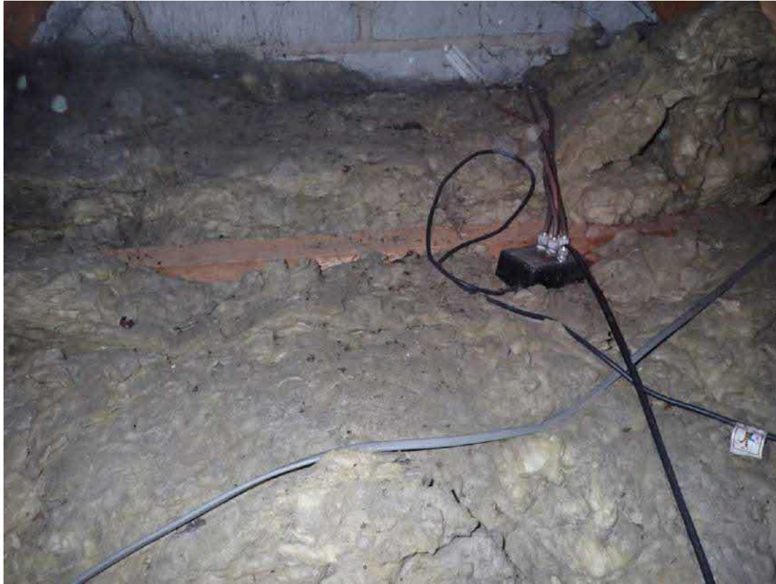
Photograph 11 – thick loft insulation and evidence of cluster flies.
