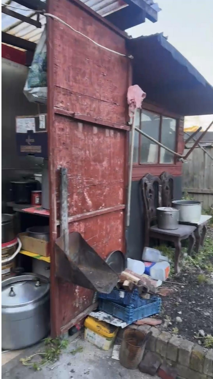
Photo 2: Shed B with rotten wooden wall and door with broken windows
