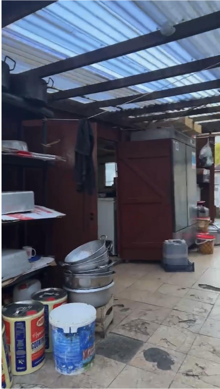
Photo 3: The fractured floor tiles and plastic ceiling cover
