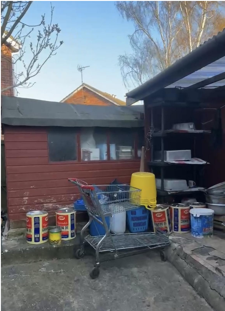
Photo 1: Shed A with rotten wooden wall and cracked ceiling roof
