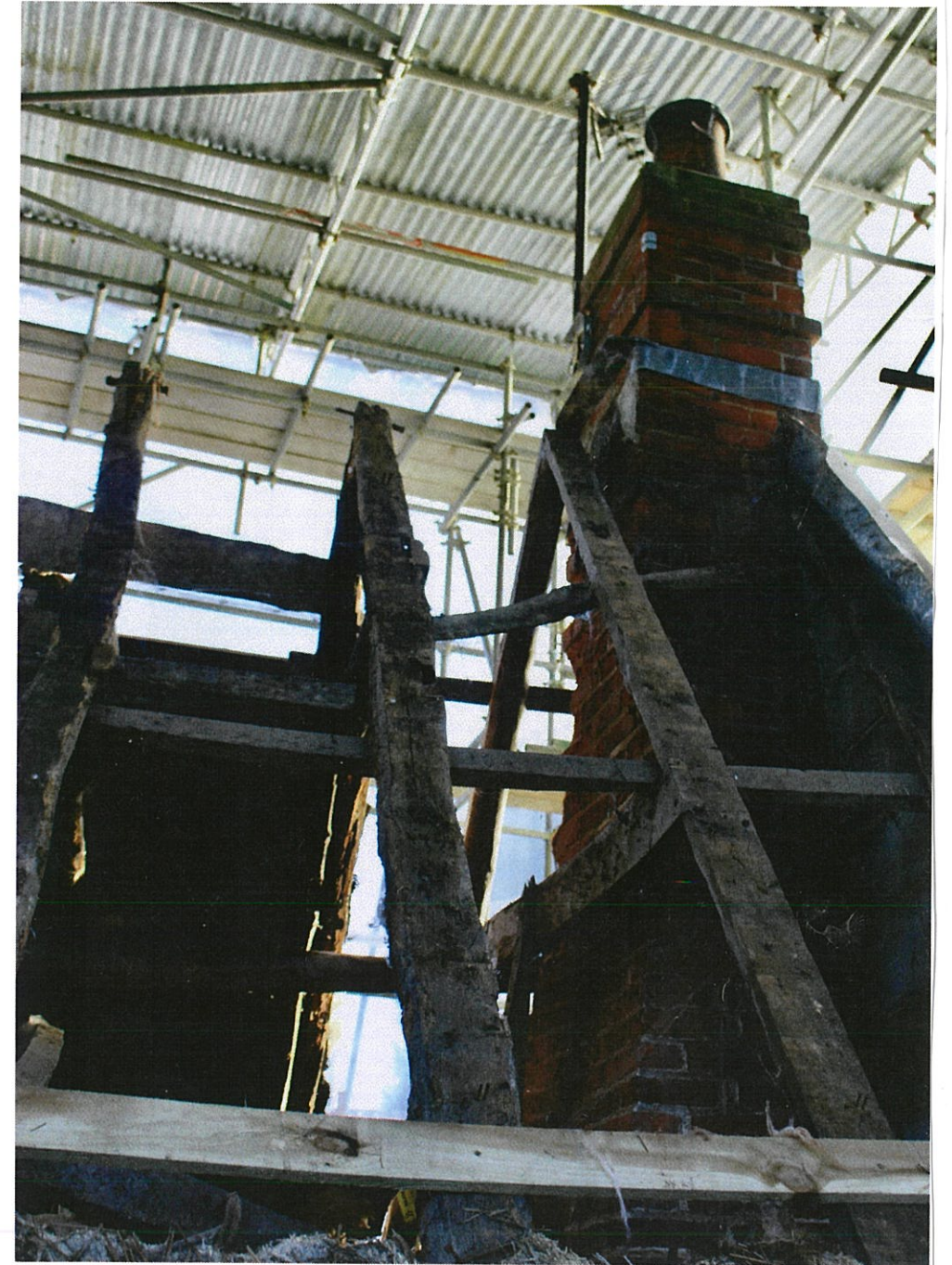
• BRICK CHIMNEYS NEED REPAIR TO ERODED BRICKS & CRACKS & TIEING TO ROOF STRUCTURE
