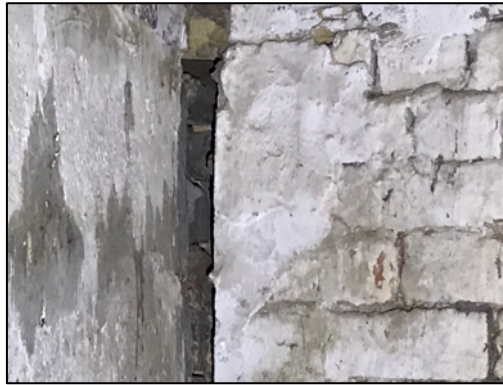
Figure 17 – crevices in the brickwork on the eastern end of the stables
