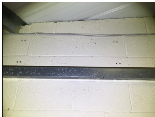
Figure 11 - gaps above the wall plate within the warehouse with pipistrelle droppings
