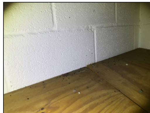
Figure 12 – hundreds of pipistrelle type droppings within the warehouse
