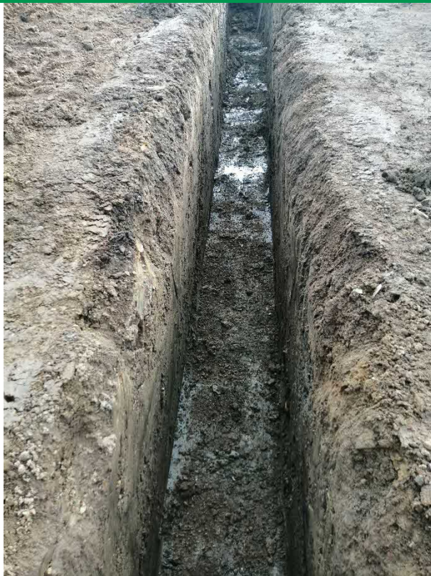
PLATE 4 – 19.01.23 INSPECTION OF FOUNDATION TRENCHES WITHIN WESTERN SITE AREA PRIOR TO CONCRETE POUR
