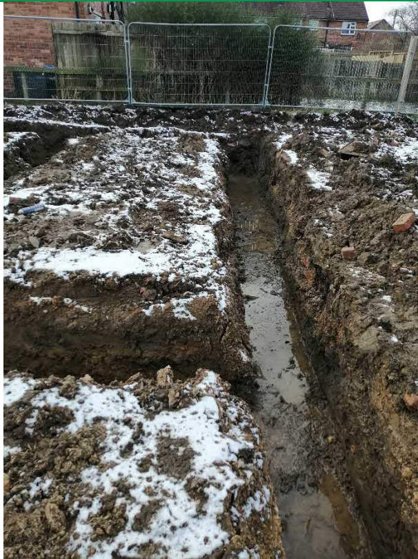
PLATE 3 – 19.01.23 INSPECTION OF FOUNDATION TRENCHES WITHIN WESTERN SITE AREA PRIOR TO CONCRETE POUR
