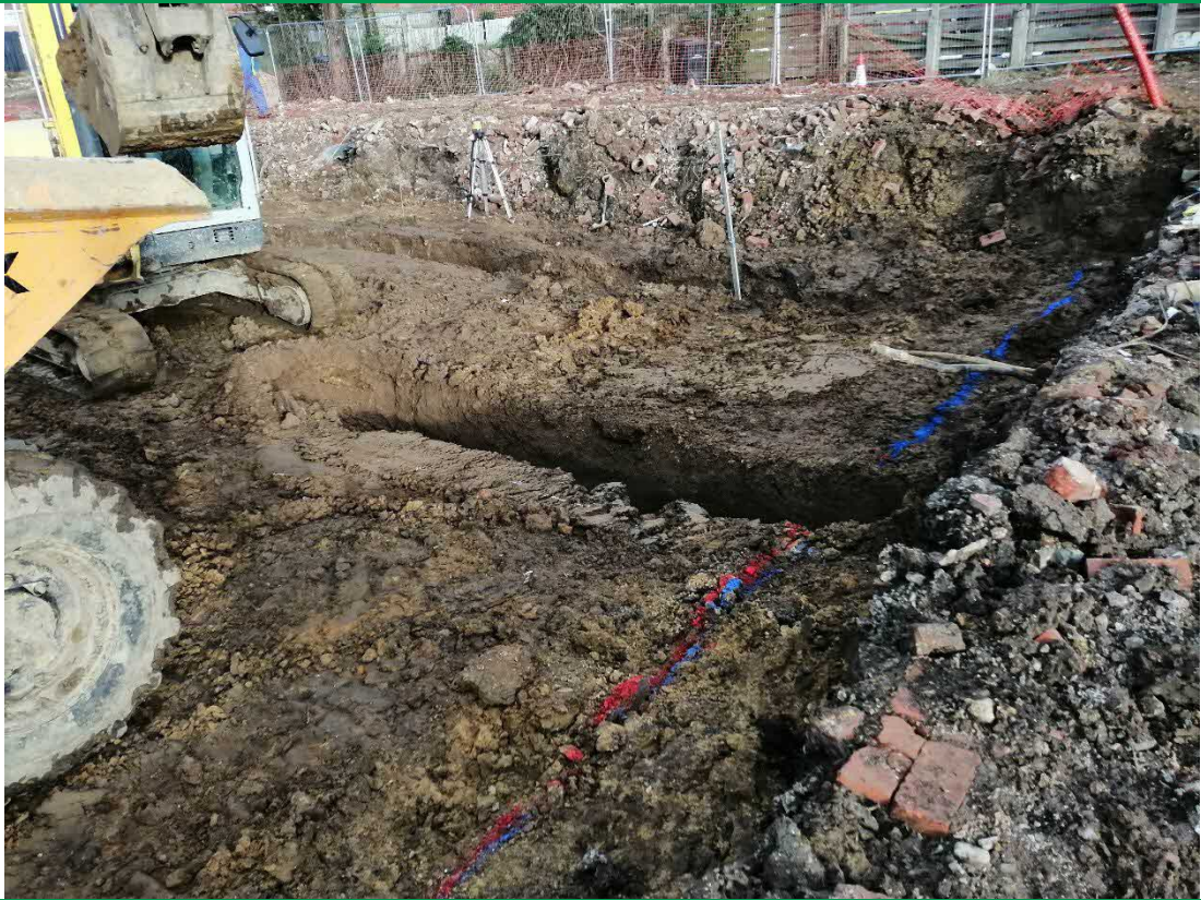
PLATE 3 – SHOWING GENERAL REDUCTION IN LEVEL. THOUGH ALSO SHOWING BUILD UP OF HAUL ROAD
