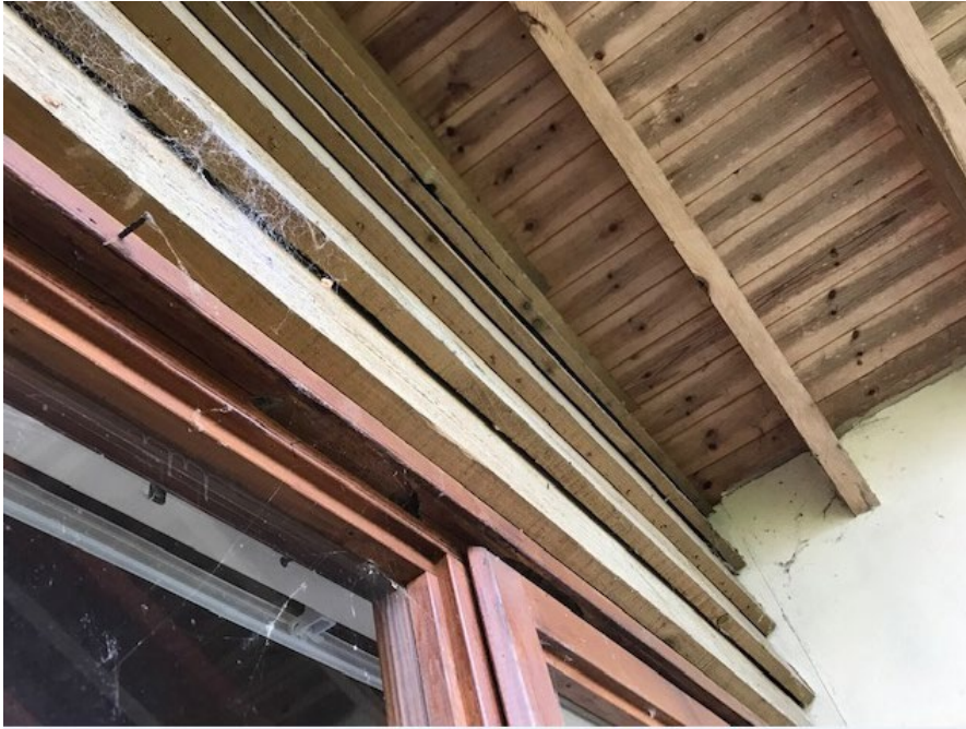
Cladding within balcony showing gaps beneath timbers (2018)
