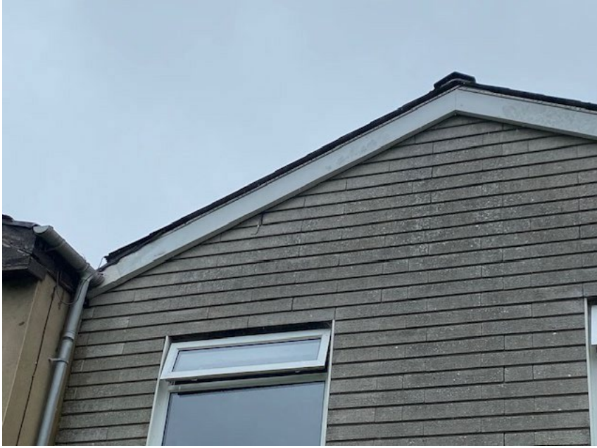
Small gap to loft noted in cladding below bargeboard over centre of window on south-east front gable (2023)
