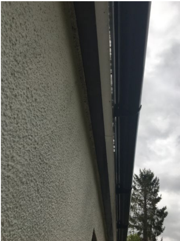
Tight fascia on front south-east elevation (2018)
