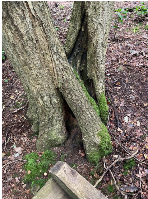
Photograph 4: T1442 oak with decay and twin stems leaning over track.
