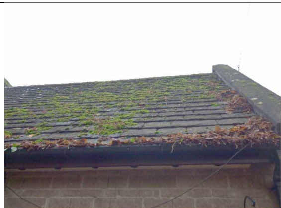
Photo 2: Roof tiles were found to be tightly overlapped.
