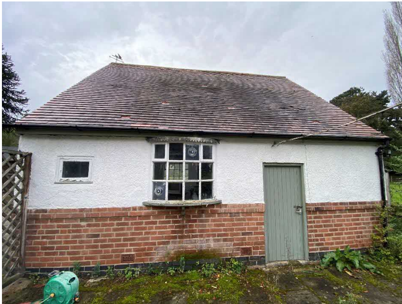
Southern aspect of B2 showing some missing tiles
