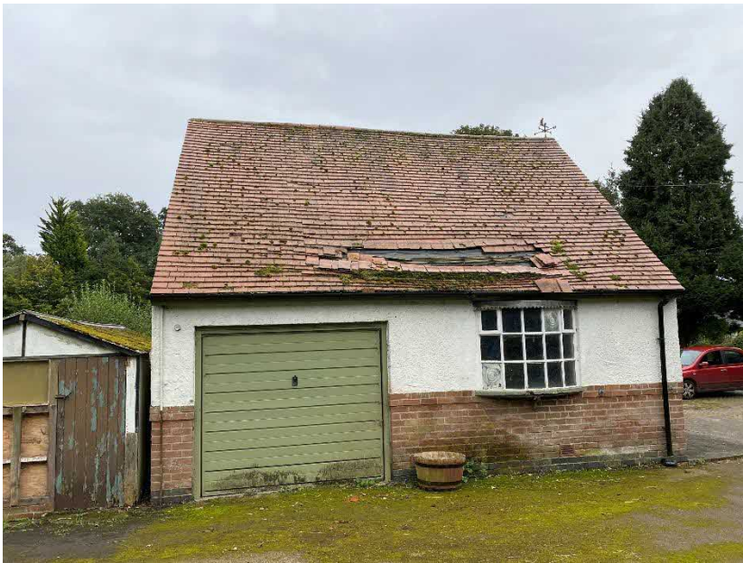
Northern aspect of B2 and B2a showing the large area of slipped and missing roof tiles
