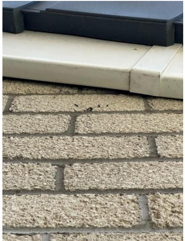
Photo 2 – Bat droppings found below lifted fascia cover on B1
