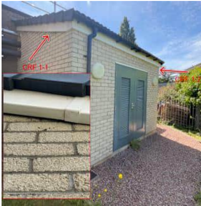
Photo 1 – B1 Confirmed roost and bat droppings (north and south elevations)
