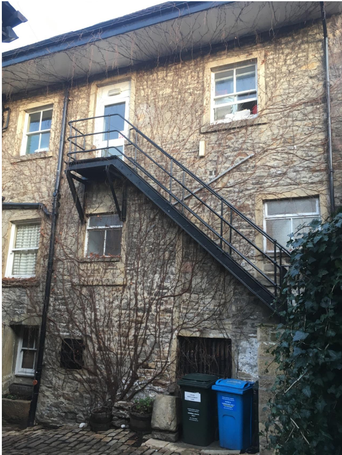
Figure 10: rear elevation showing 2no partially blocked up windows and new fire escape. Note the irregular pattern of the door and window opening in contrast to the road facing elevations.
