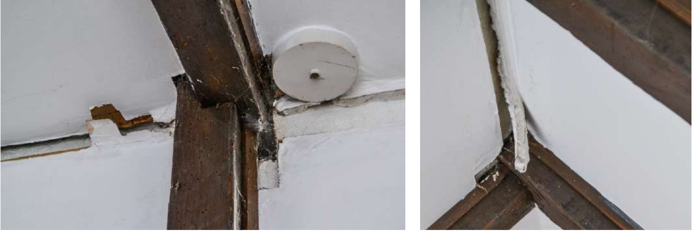
30. Signs of Movements in Roof Structure
