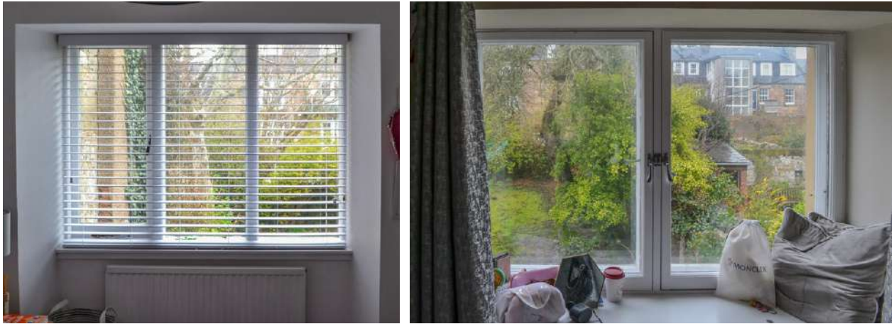
21. Modern timber casement windows - non original openings - no recorded permission
