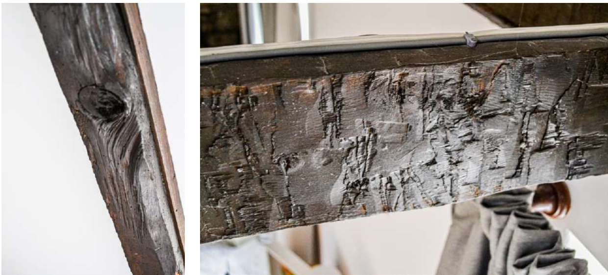
27. Texture disparity between original timber structure (left) and decorative joist (right)
