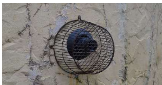
Flue installed as part of the approved application 02/02660/EFULL in 2002.
