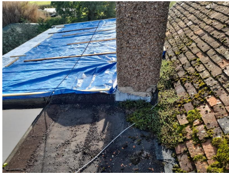
Photograph 2 Main flat roof to first floor has been covered with a tarpaulin as a temporary measure to prevent further water ingress
