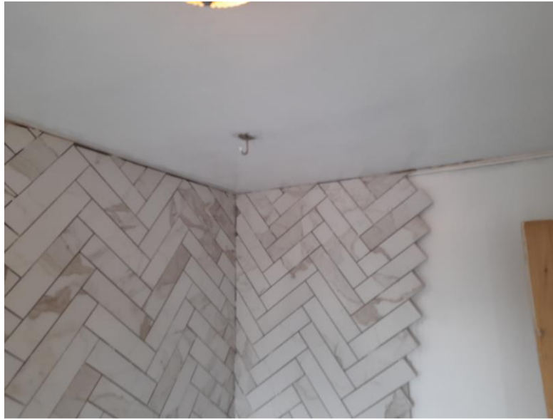
Photograph 10 Water ingress around ceiling has prevented completion of tiling to Bathroom
