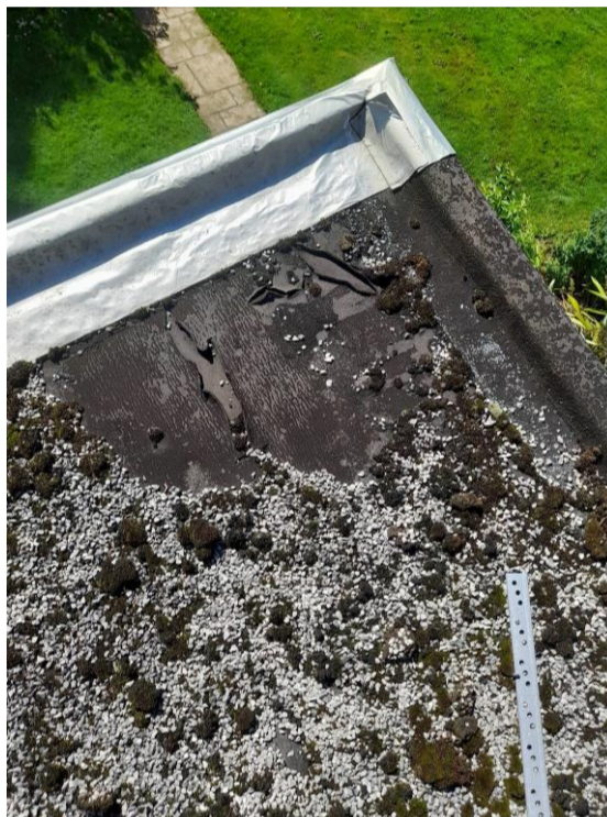
Photograph 13 Previous flashband repairs above first floor Ensuite Bathroom, with wide splits in bitumen directly in front
