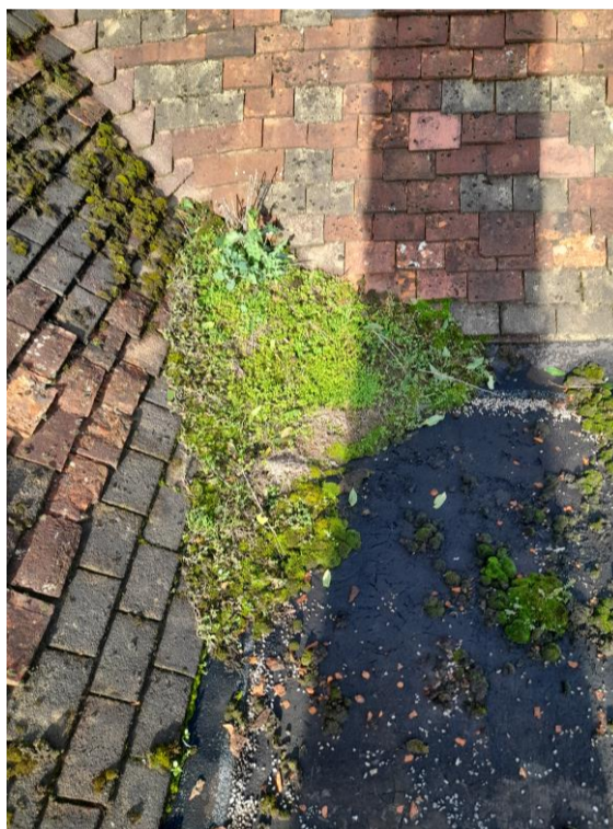
Photograph 11 Longstanding lack of maintenance to flat roof over two storey rear entrance has caused significant water damage to Landing underneath
