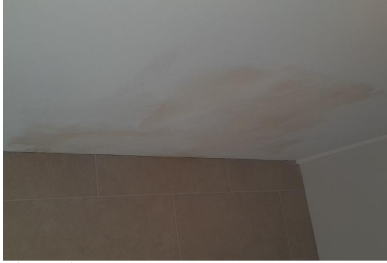
Photograph 18 Further damage to opposite side of first floor Landing ceiling
