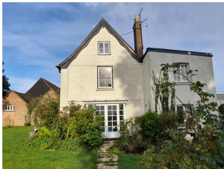
Photograph 5 View of South East side elevation showing flat roof to two storey extension
