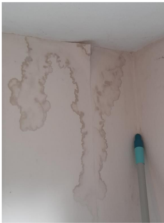
Photograph 8 Longstanding damp patches to entrance Corridor
