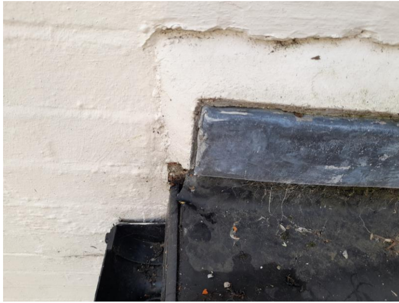
Photograph 7 Close up of corner of roof above back door, with open joints causing water ingress
