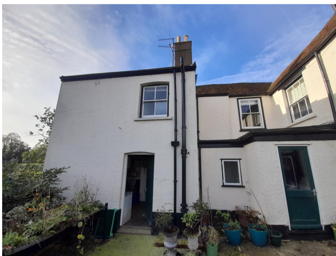
Photograph 1 Rear elevation of Pursley Farmhouse showing flat roofs in need of urgent repair
