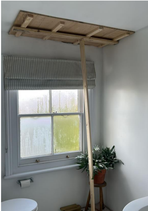
Photograph 15 Temporary support to collapsing ceiling in Landing Bathroom
