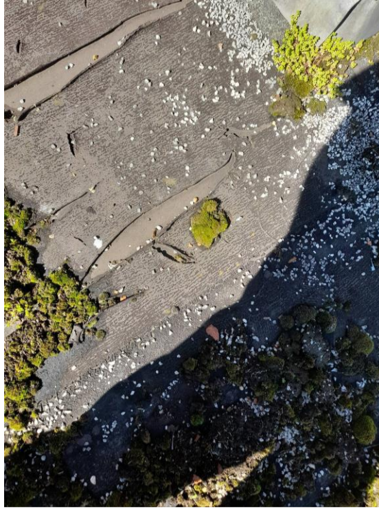
Photograph 12 Wide splits to bitumen are evident in many places on two storey extension
