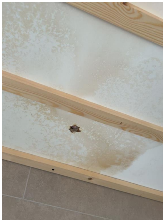
Photograph 16 Puncture hole in Ensuite Bathroom ceiling to release water & prevent collapse
