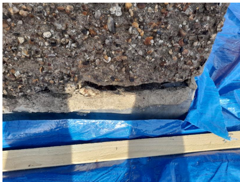
Photograph 14 Open junction to base of chimney to two storey extension, enabling direct water penetration
