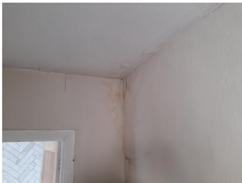
Photograph 9 Water staining & mould to corner of Bathroom
