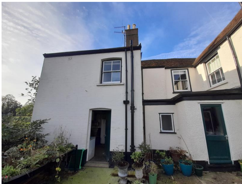
Side elevation of Pursley Farmhouse showing flat roofs in need of urgent repair
