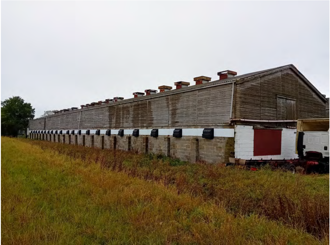
Photograph 15: Shed 1 at the southern end of the site. Viewed from southern boundary. Surface water ditch in foreground.
