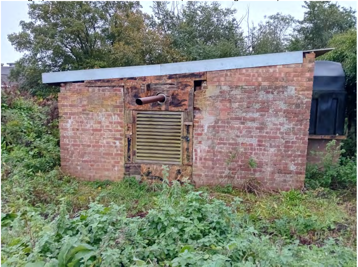
Photograph 4: Generator building south west corner. Above ground bunded tank to the right.
