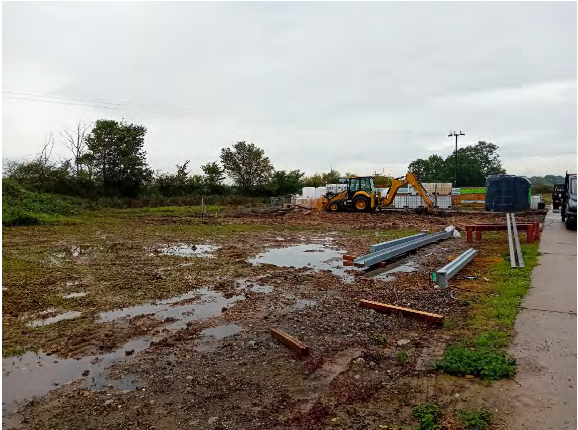
Photograph 1: Western side of the site where the new building is proposed. Bunded diesel tank on the right hand side.
