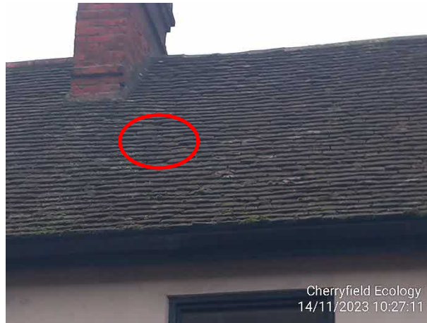
Figure 7: Examples of gaps present in B1
