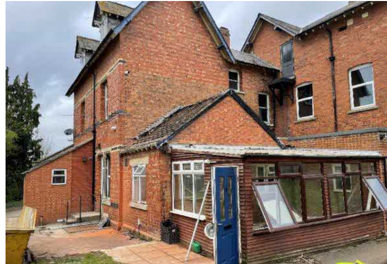
Plate 19: Former Conservatory style building and brick extension on the southeast elevation as seen in March 2023, now removed.
