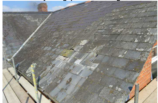
Photograph 10: Slipped tiles and gaps on northern elevation
