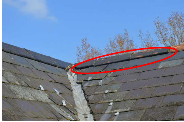
Photograph 14: Gaps under ridge tiles and slipped roof tiles
