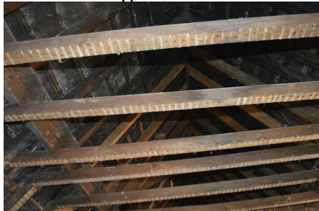
Photograph 16: Wooden rafters and roof structure with ceiling removed in north western section of the hotel
