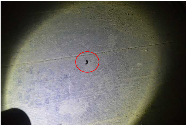
Photograph 15: Bat dropping found (BLE) in top floor room in SW section
