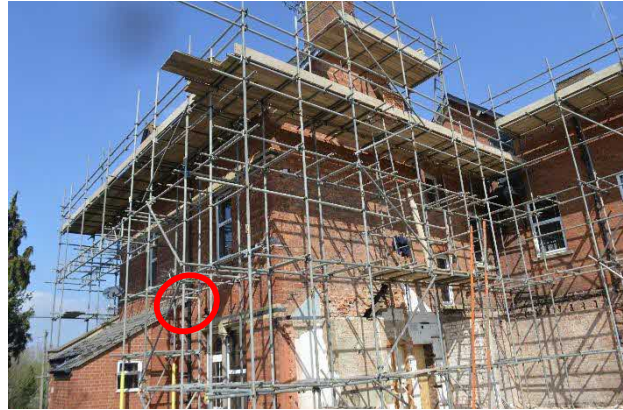
Photograph 2: S elevation – Location of emergence and return of bat to roost (EM2, RE2)
