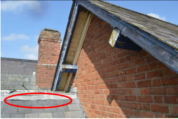
Photograph 13: Gaps under lifting lead flashing
