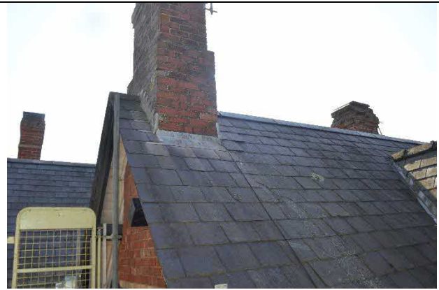
Photograph 8: N elevation gable features near chimney and gaps beneath ridge tiles
