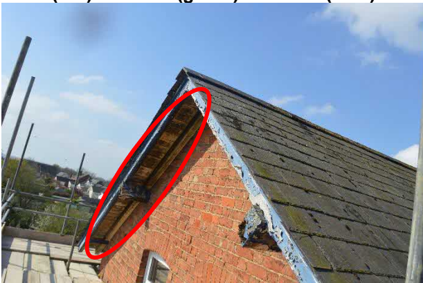
Photograph 11: Gaps on gable end on eastern elevation – most likely bat access point beneath the barge board (for the Whiskered and common pipistrelle maternity roosts) due to staining (suspected fur staining) present between the barge board and the brickwork
