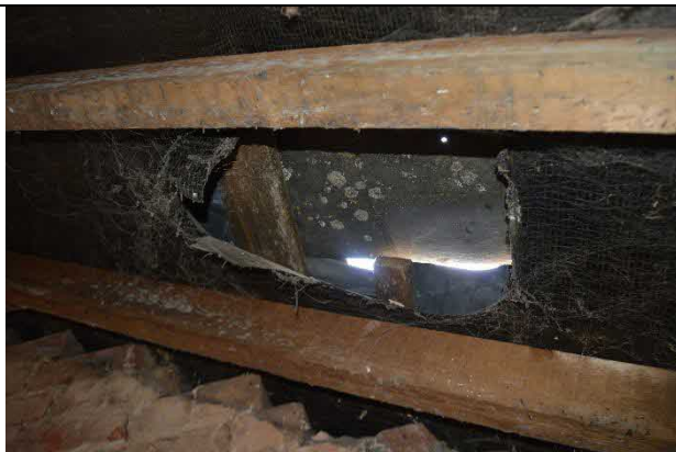
Photograph 22: Large hole in bitumen felt
