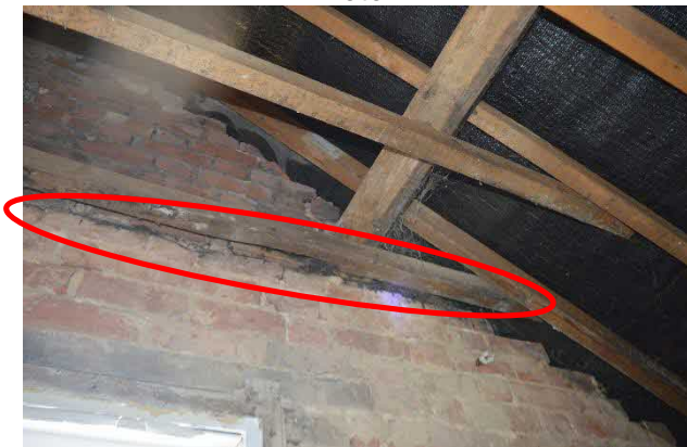
Photograph 19: Exposed void near E gable and large accumulation of droppings between joist and the brickwork (circled)
