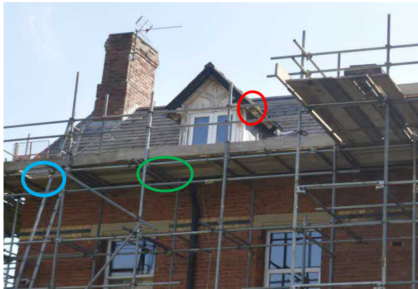
Photograph 9: W elevation - Location of EM1 (red) and RE1 (green) and EM3 (blue)
