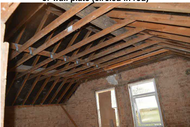
Photograph 23: Exposed rafters in south western section of the hotel
