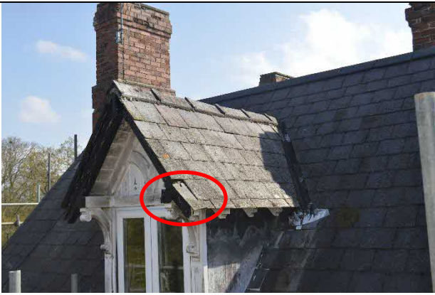
Photograph 7: Slipped tiles on dormer window on western elevation where EM1 located
