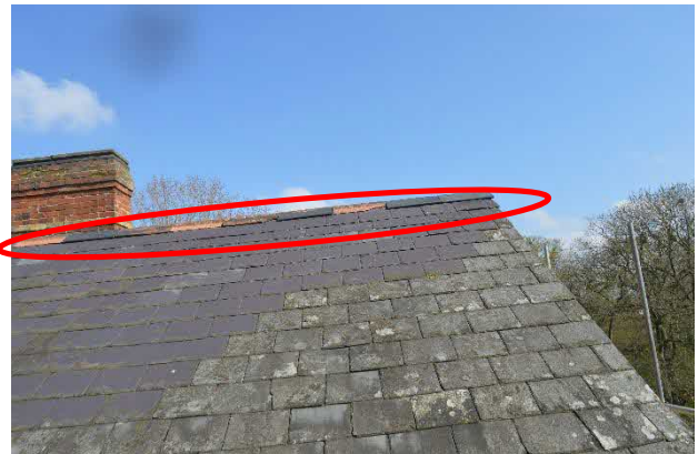
Photograph 12: Gaps under ridge tiles near eastern gable end
