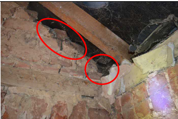
Photograph 21: Large holes and cracks in brickwork and large pile of bat dropping on to or wall plate (circled in red)
