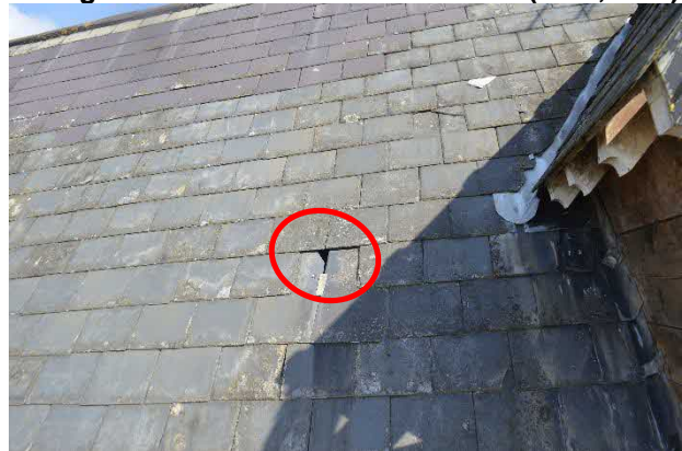
Photograph 4: Slipped tiles and gaps on southern elevation
