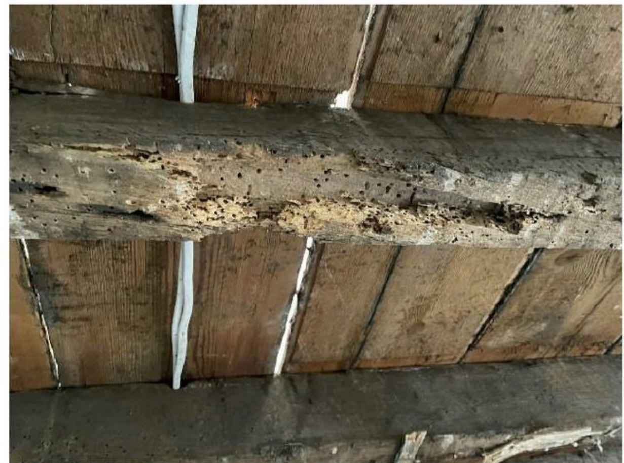
Figure 16 – Joist d 9, significant loss to central underside to 1/3 depth
