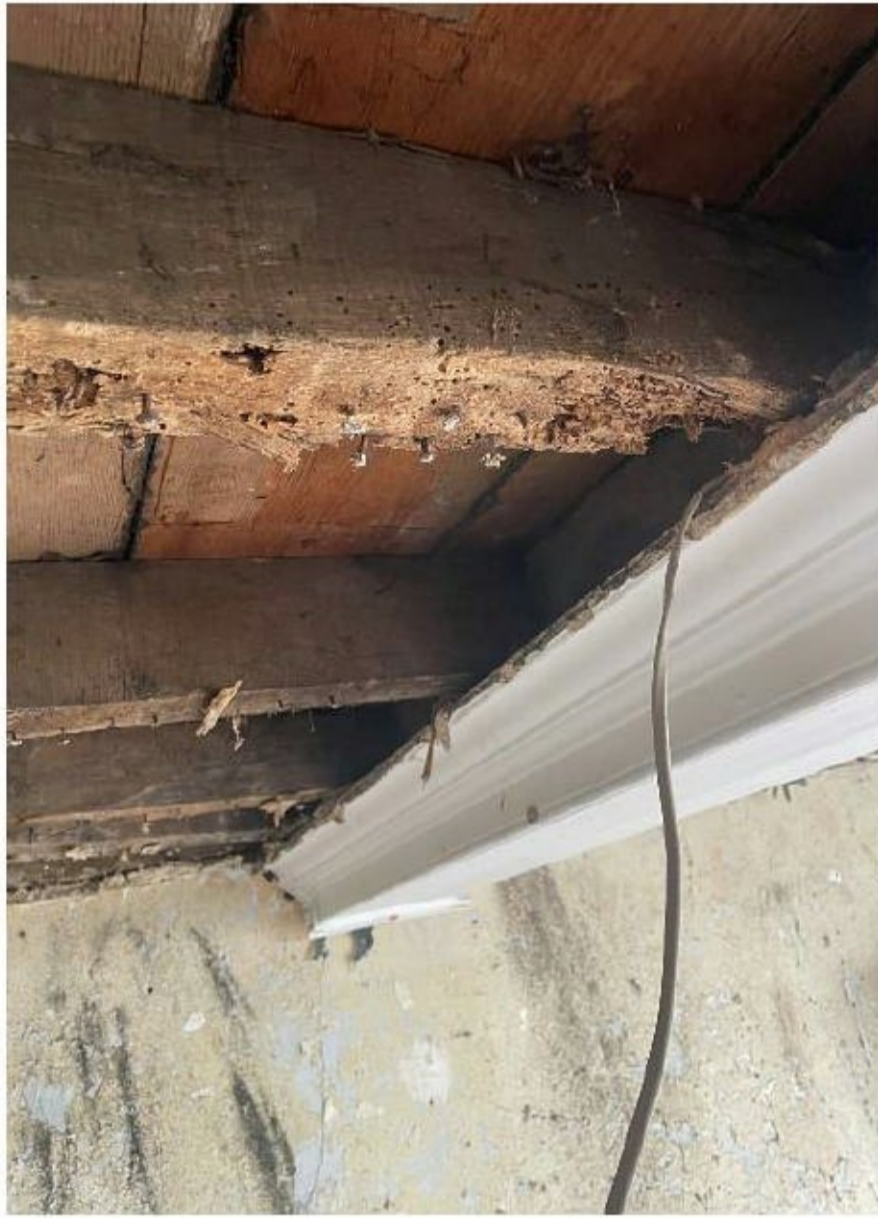
Figure 12 – Joist b 4, loss of material to ½ joist depth
