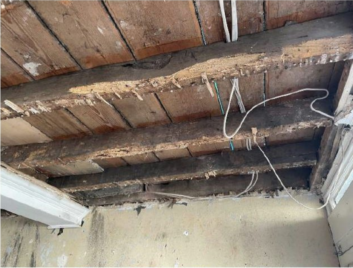
Figure 8 - View of joists a:1-4, note material loss to underside of 3 & 4
