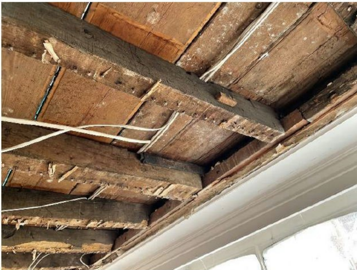
Figure 4 - View of joists a:3-7, joists notched over timber batten. Note metal strap to side of wider joist 6.
