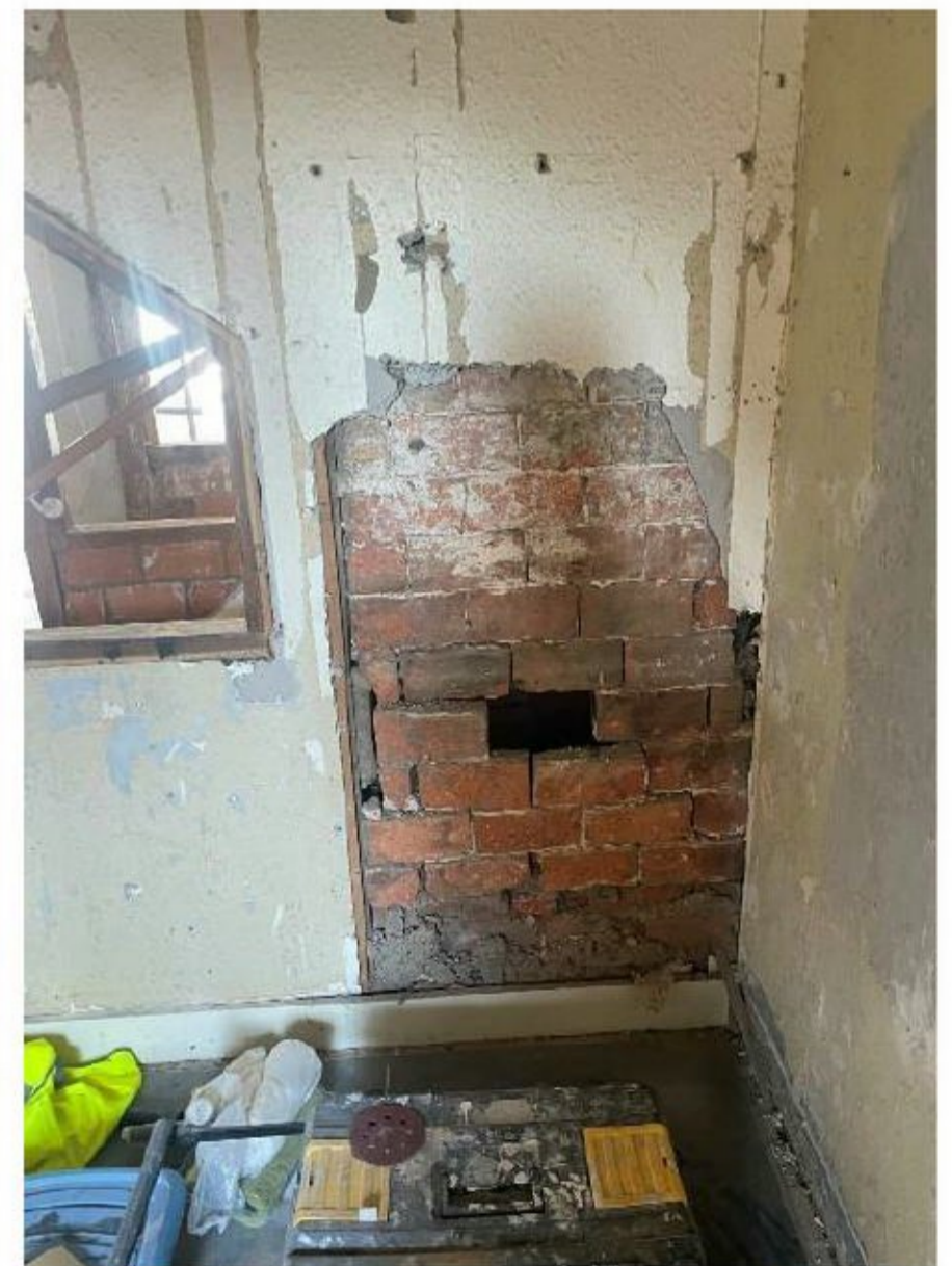
Figure 19 - Southern wall with unstable masonry panel
