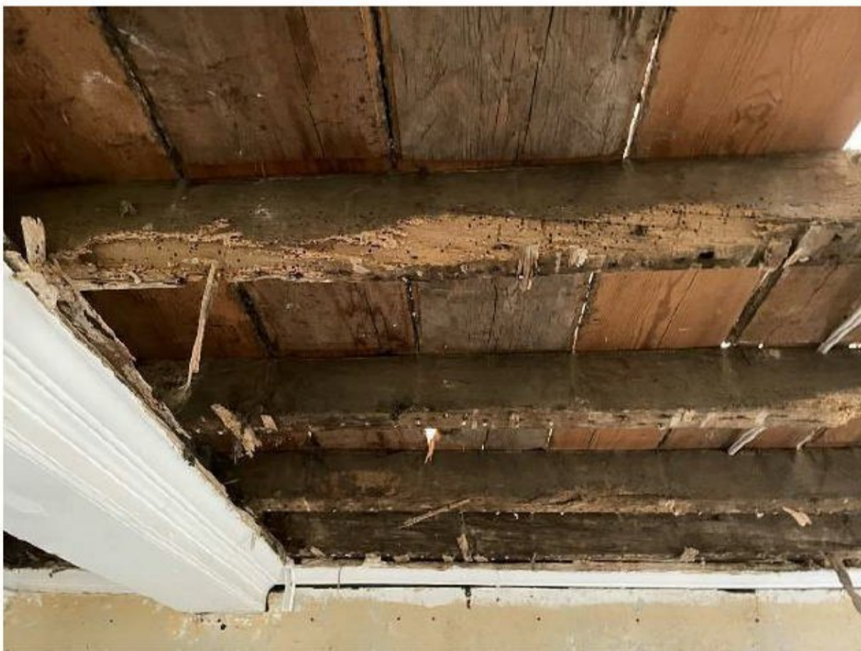
Figure 15 – Joist d 8, significant loss of material to north end west side
