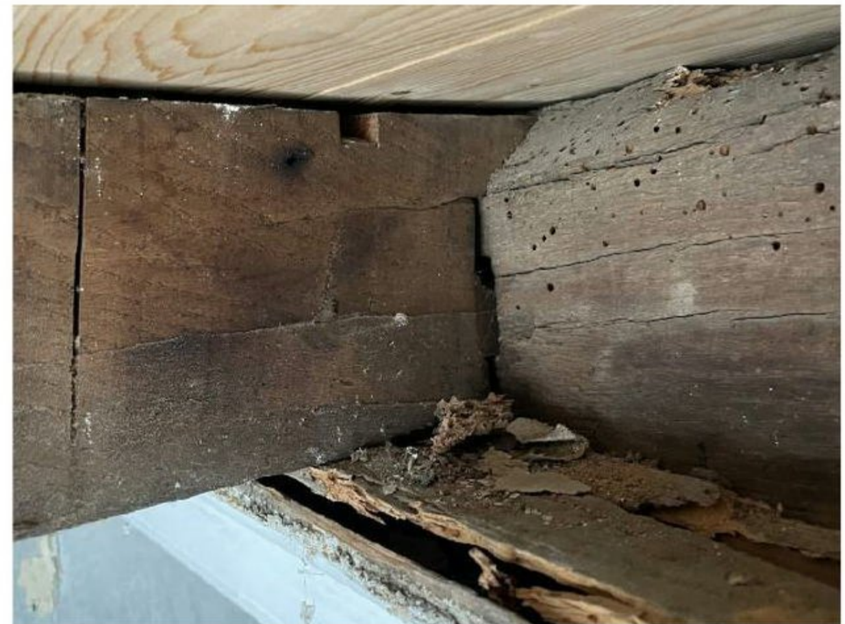
Figure 5 - Typical joist notching into primary beam A, some flight holes in side of beam
