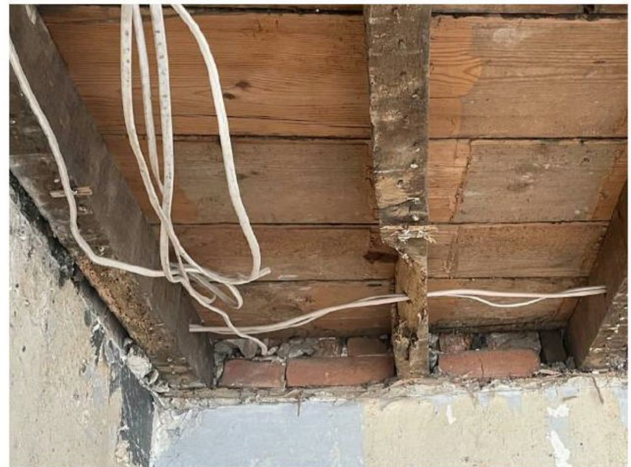
Figure 11 – Joists b 10 & 11, south bearings. Significant loss to joist 10.
