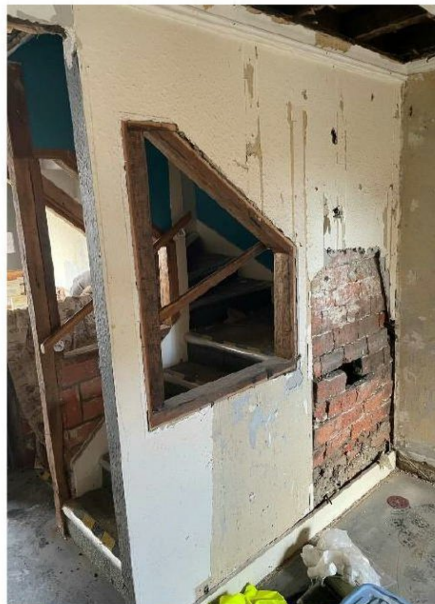
Figure 18 – Southern wall with unstable masonry panel
