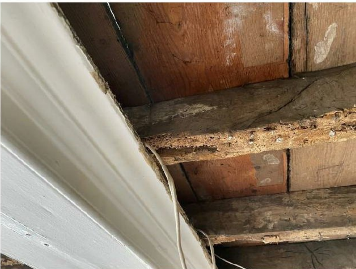
Figure 10 – Joist b 4, loss of material to \frac{1}{2} joist depth
