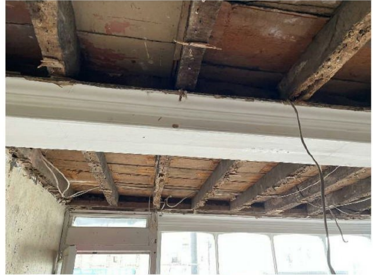
Figure 9 - View looking north from bay b to a, beam A with decorative mouldings in place.
