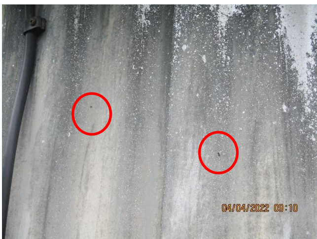
Photo 16: Bat droppings on external of 'B2'.
