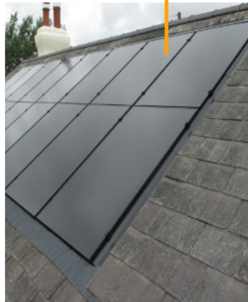
Solar Photo voltaics in roof
